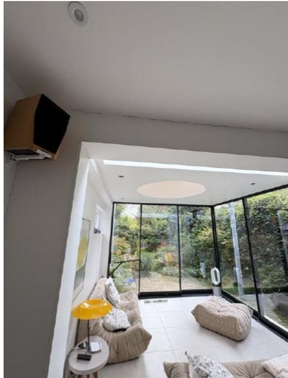
Cracking about support beam.
