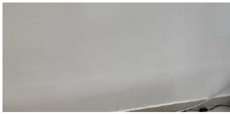
Cracking to extension wall
