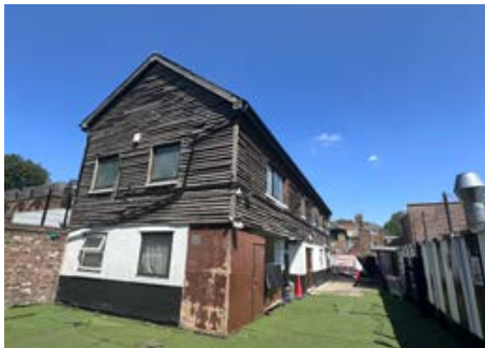
Figure 5.14 Southern elevation of the extension built in 2004 showing later UPVC window (ground floor) and ply wood (ground floor corner). Source: Author [Dated: 25.07.2025]
