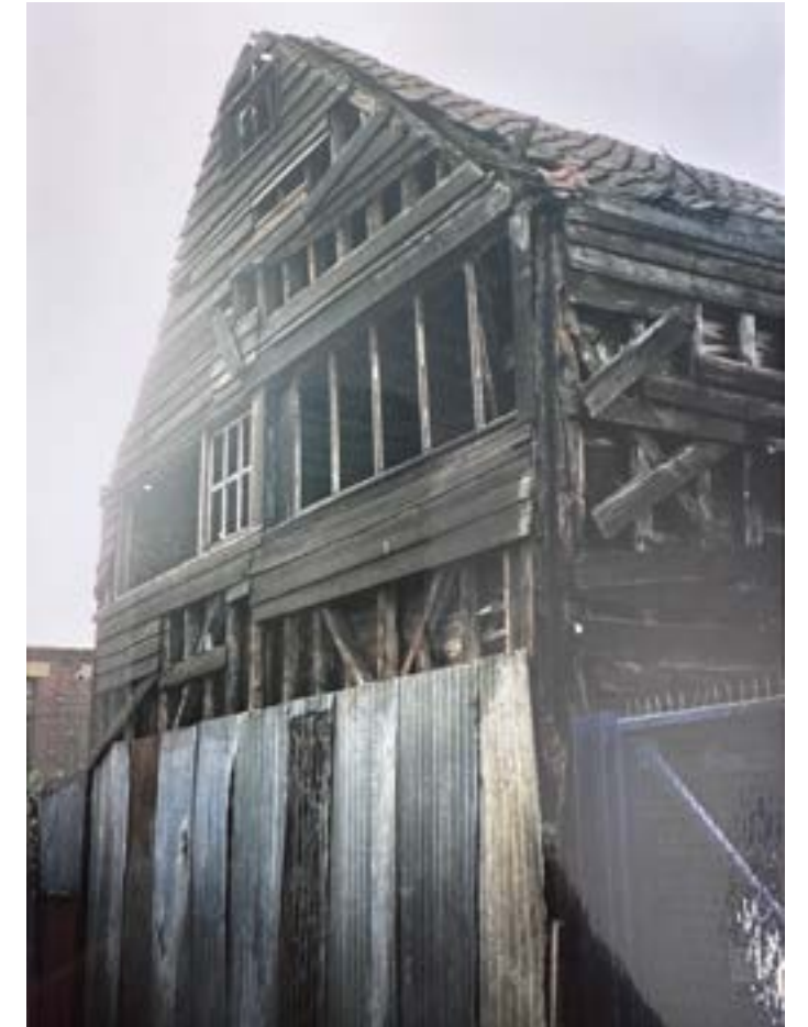
Figure 4.22 Photo of eastern elevation, 1999, in dilapidated condition. Source: Bruce Castle Museum
