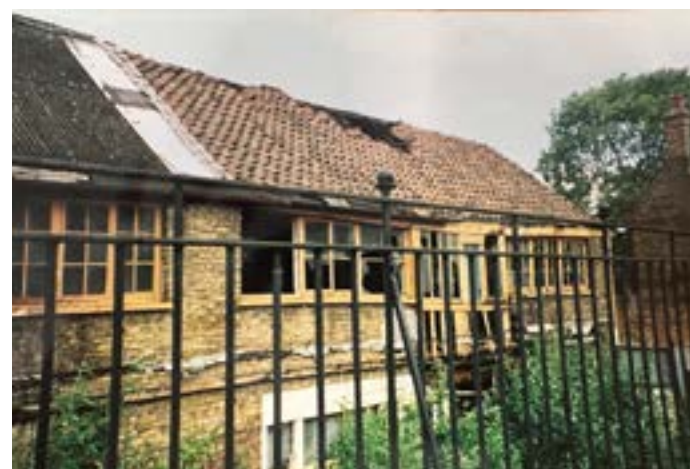
Figure 4.21 Photo of the western elevation taken in 1999, in dilapidated condition. The far side in tile roof is the 18th C part of the Barn Source: Bruce Castle Museum
