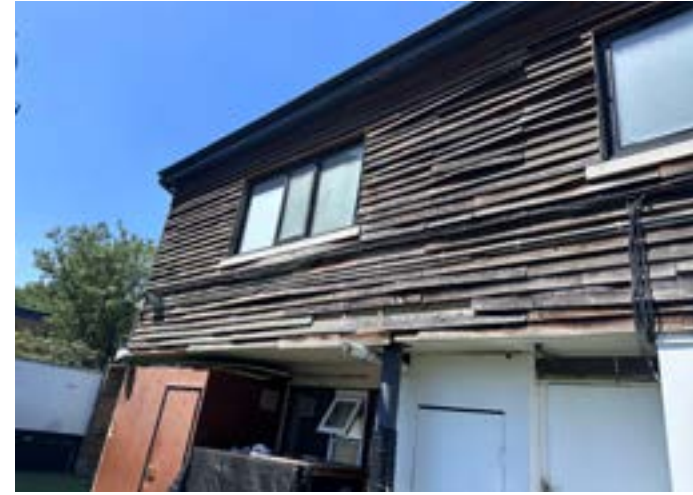
Figure 5.15 Eastern corner of the 2004 office extension, showing later ad hoc insertion of plywood and the poor quality of the timber cladding. Source: Author [Dated: 25.07.2025]
