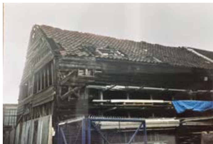
Figure 4.20 Comparative photo of the northern and eastern elevation taken in 1999, in dilapidated condition. Source: Bruce Castle Museum
