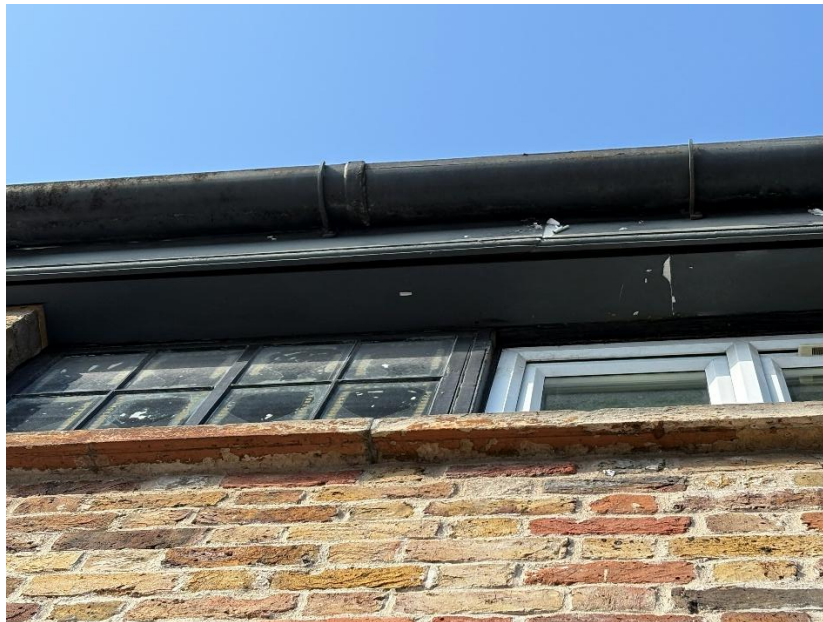
Image 11 – Gap between soffit and fascia of B2 (Aval Consulting, 2026)
