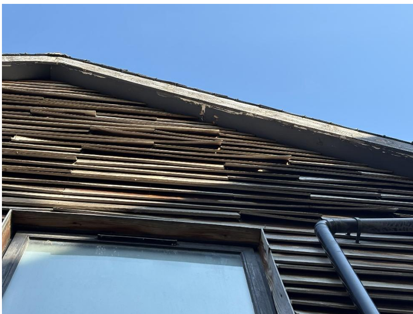
Image 10 – Gaps along the south side of B1 (Aval Consulting, 2026)
