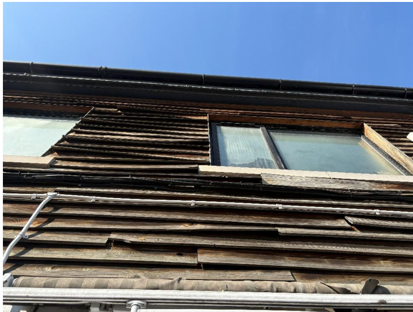
Image 9 – Gaps along west side of B1 (Aval Consulting, 2026)
