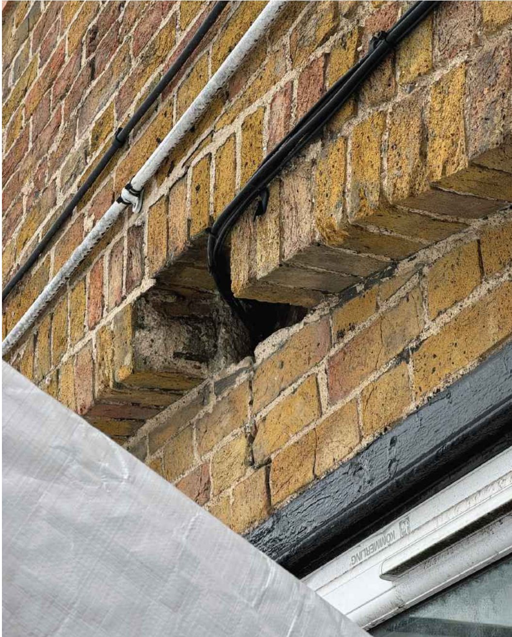
Photo 14 - East Elevation - Damage to Brickwork Arch
