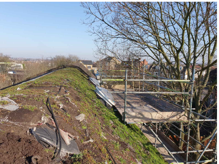
DEFECTIVE EXISTING ROOF FINISH
