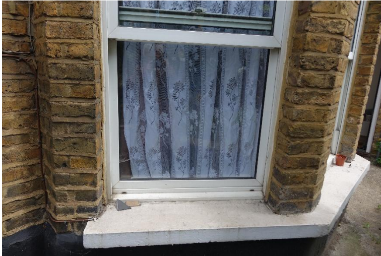
Photo 2: Front Bay Window
