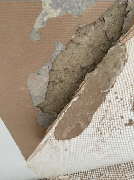
Lime plaster behind gypsum with face coming off during removal
