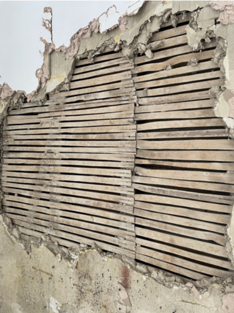
Existing laths behind areas of cracked or blown lime plaster
