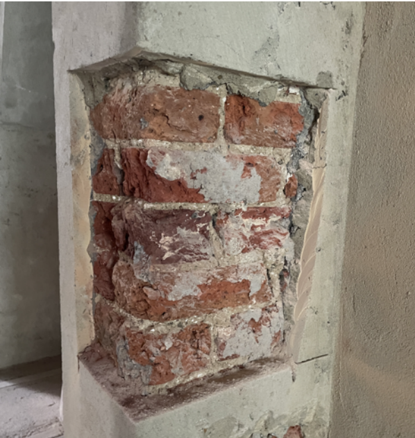
N1 - Chimneybreast corner trial area to northern wall with extensive damage. Almost all the brick faces are coming away. Bricks remain stable, but render removal over corner is more difficult and thin pier is venerable. Render to remain in place.
