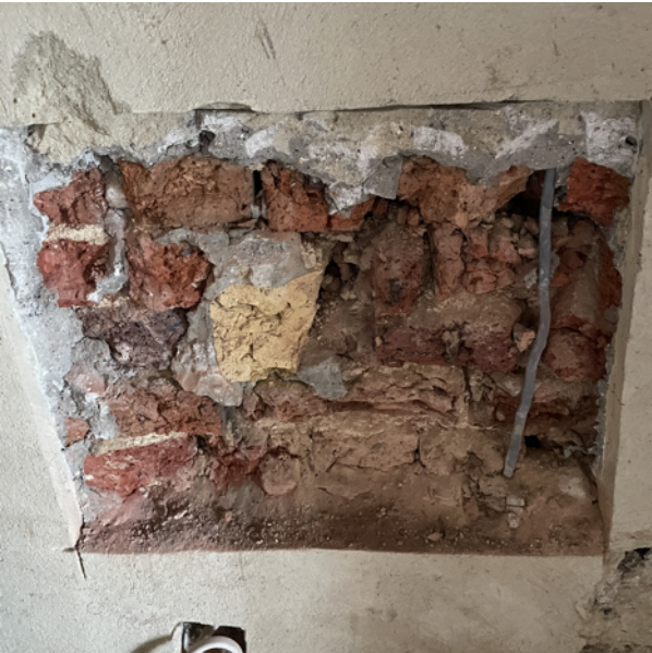
N4 - Chimney back trial area to northern wall with extensive damage. Brick faces are coming away bricks are crumbling with large chunks falling away. Render to remain in place over chimneybreasts.
