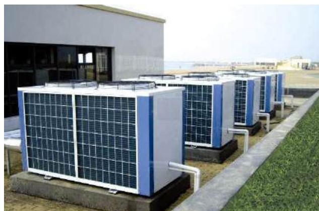
Figure 6: Outdoor ASHP units.
