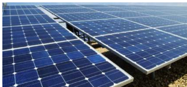
Figure 4: Monocrystalline PV arrays
