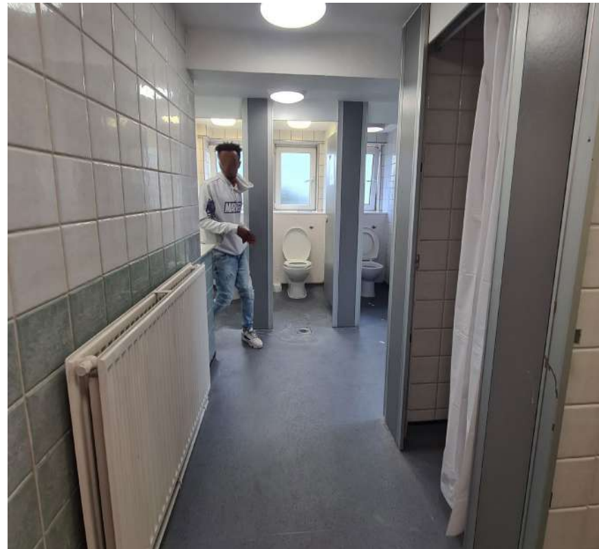
Shared WC's / bathrooms with only curtain rails providing privacy screening to shower cubicles
