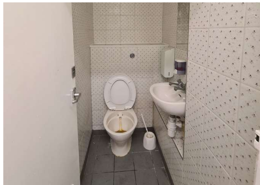
Typical shared WC
