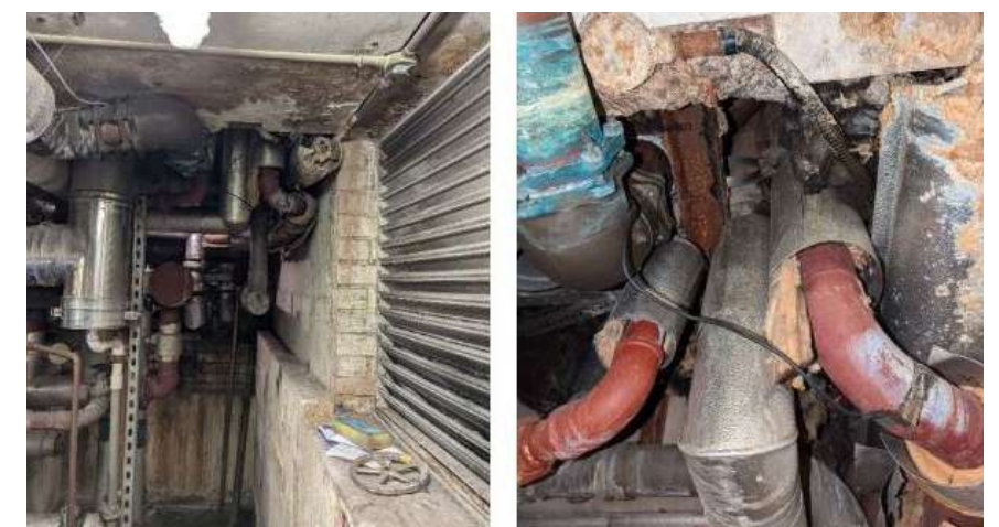
Visible damp and water ingress in basement plant / boiler room. Areas of concrete were showing signs of water damage and some visible steel members with surface rusting.
