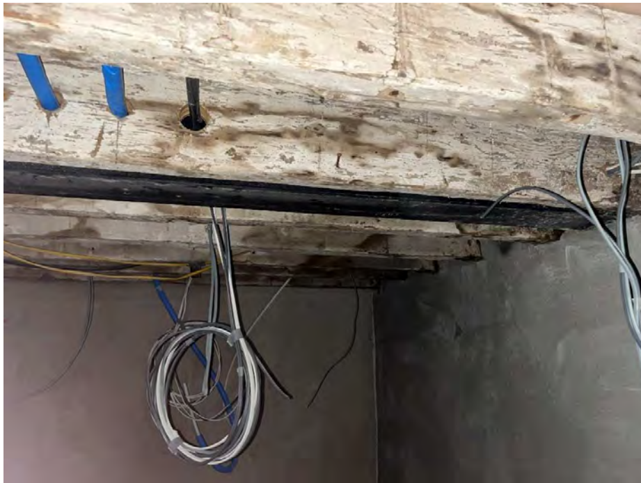
Plate 12 – Timber joists to the basement which have been altered to accommodate service runs.
