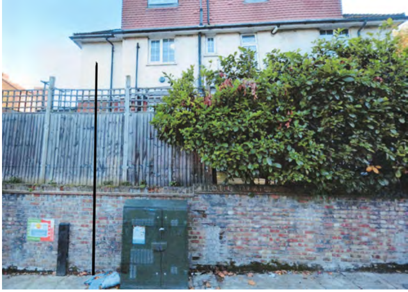
LOCATION A WITH POLE
