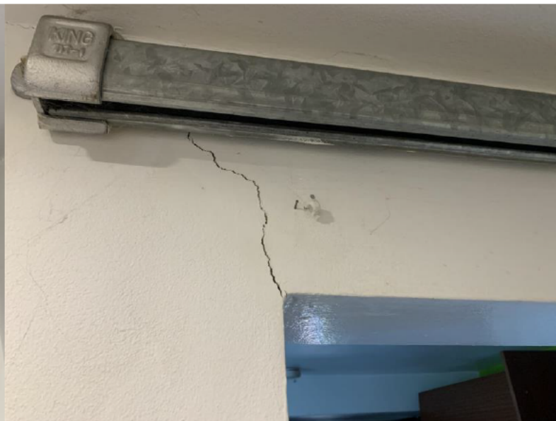
Hall - crack above kitchen door
