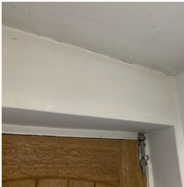
Hall - wall/ceiling cracking
