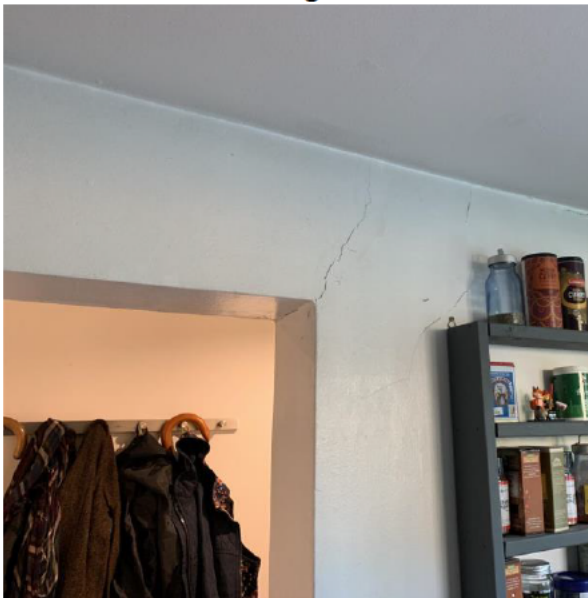
Kitchen - two cracks above door to hall
