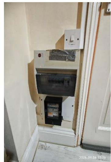
Figure 6 - Time-stamped photograph of the electricity meter serving the rear studio
