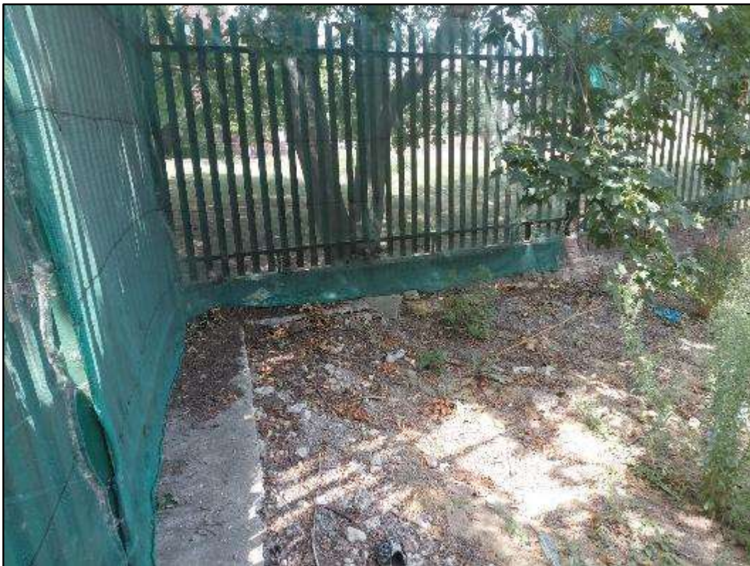
Plate 4: low wall and broken hard surfacing adjacent to T1.
