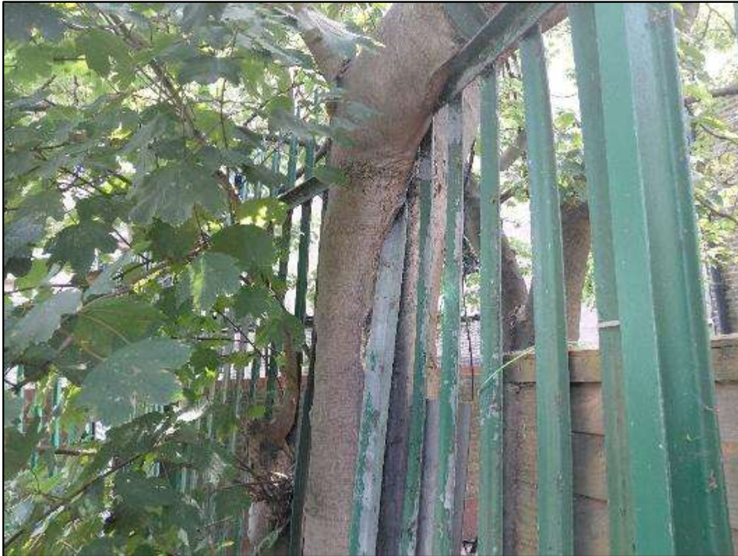
Plate 5: fencing engulfed by sycamore tree T6.
