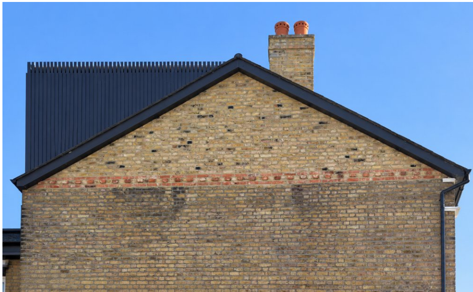
Hip to gable wall transition 12 Tancred Road, N4
