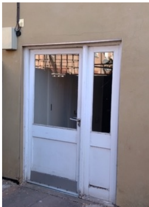
Rear Exit Door
