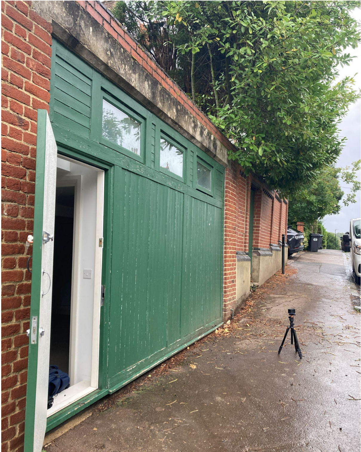
Photograph 03. Illustrating 'poor quality' workshop type appearance to front façade and access opening onto the pavement.
