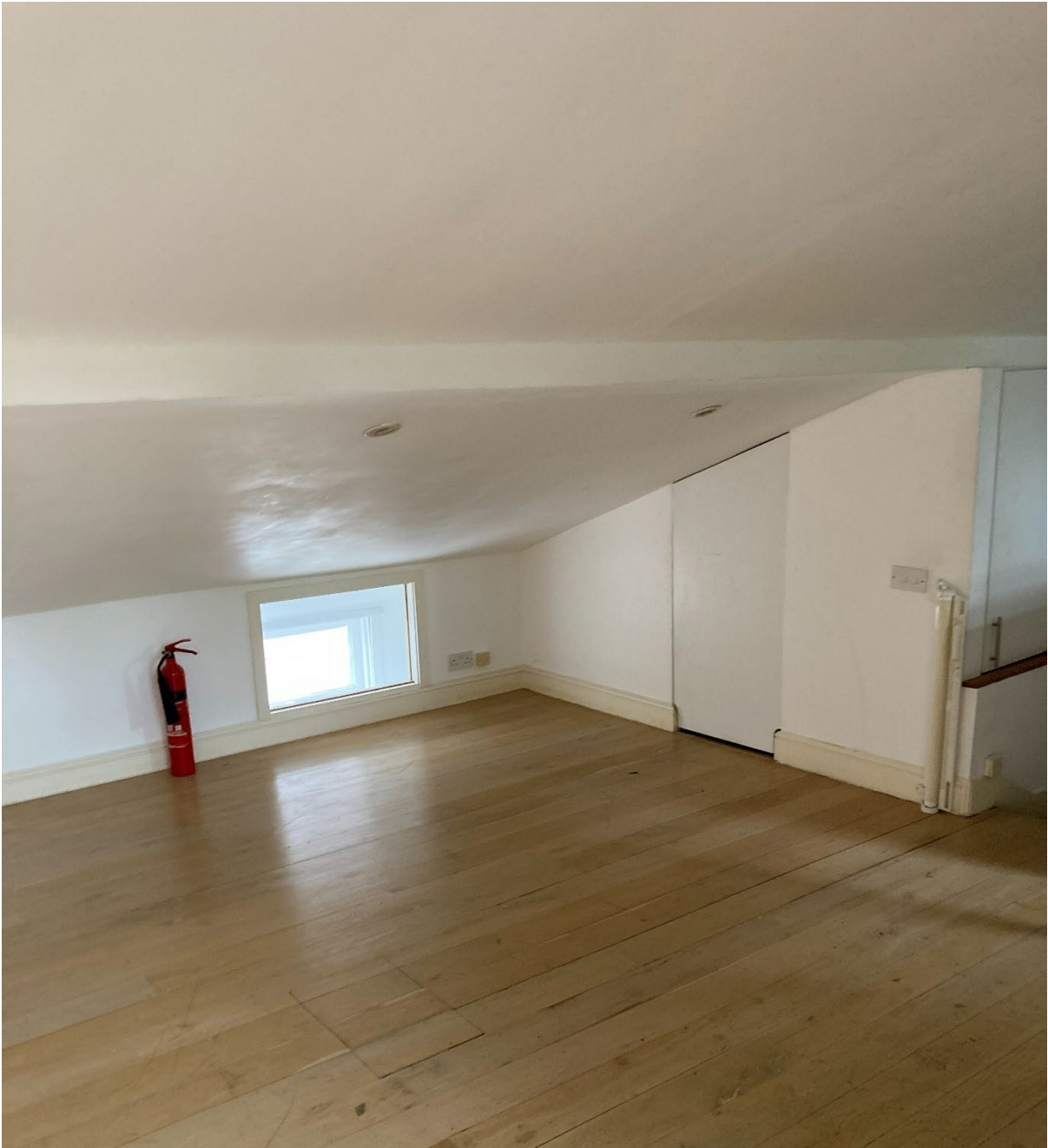
Photograph 08. Interior view illustrating how a large part of the upper floor is unusable due to very limited headroom stemming from steep monopitch roof. The addition of a roof dormer would markedly transform this space.
