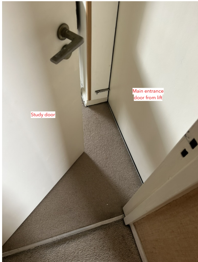
Door currently swings across Hallway in front of main entrance door
