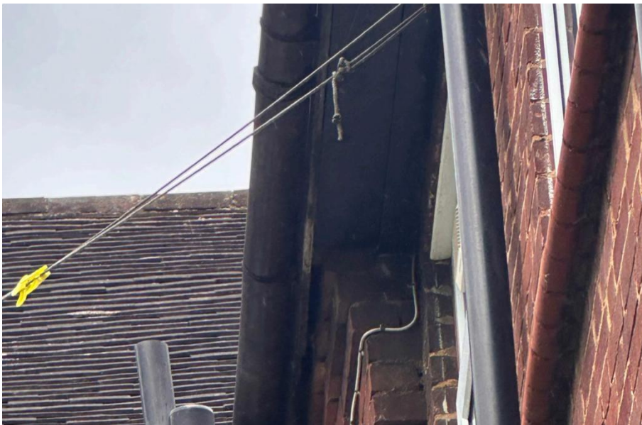
Photo 12 - Barge board gap between wall. (PRF6)
