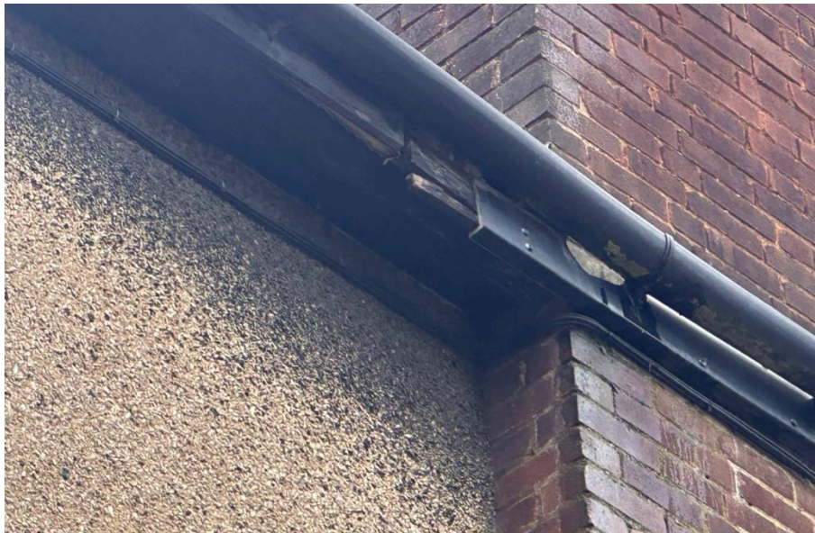
Photo 9 - Broken soffit on western aspect of the building (PRF3)
