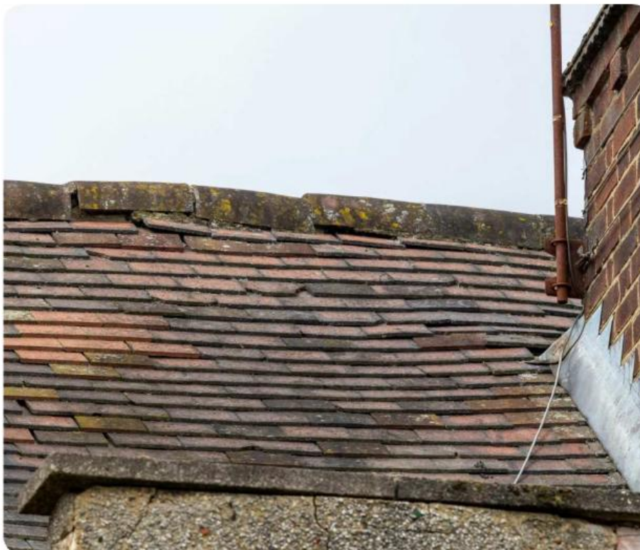
Photo 8 - Lifted lead flashing at the base of chimney. (PRF2)
