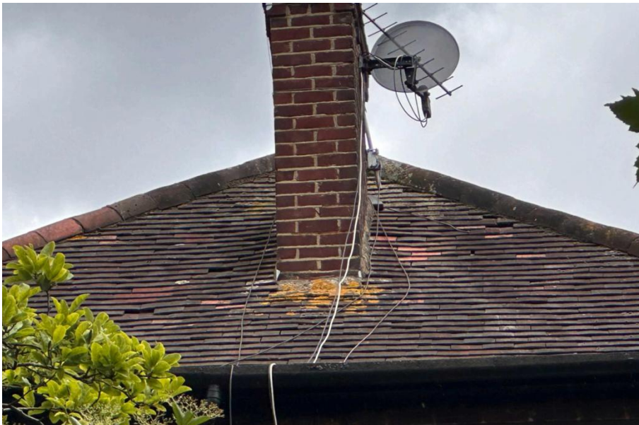
Photo 14 - Failed flashing at chimney base. (PRF8)
