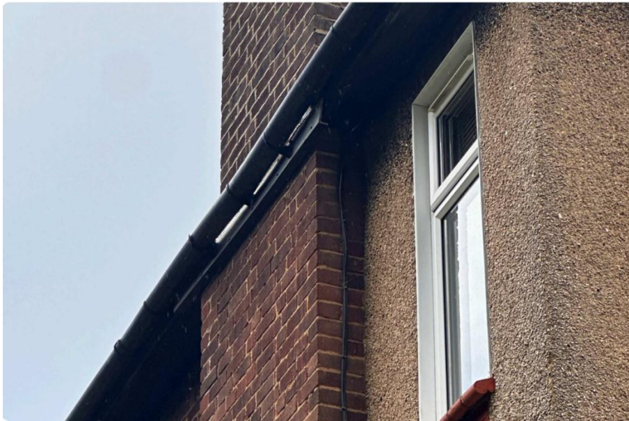
Photo 13 - Sheltered crevice between masonry and roof.(PRF7)
