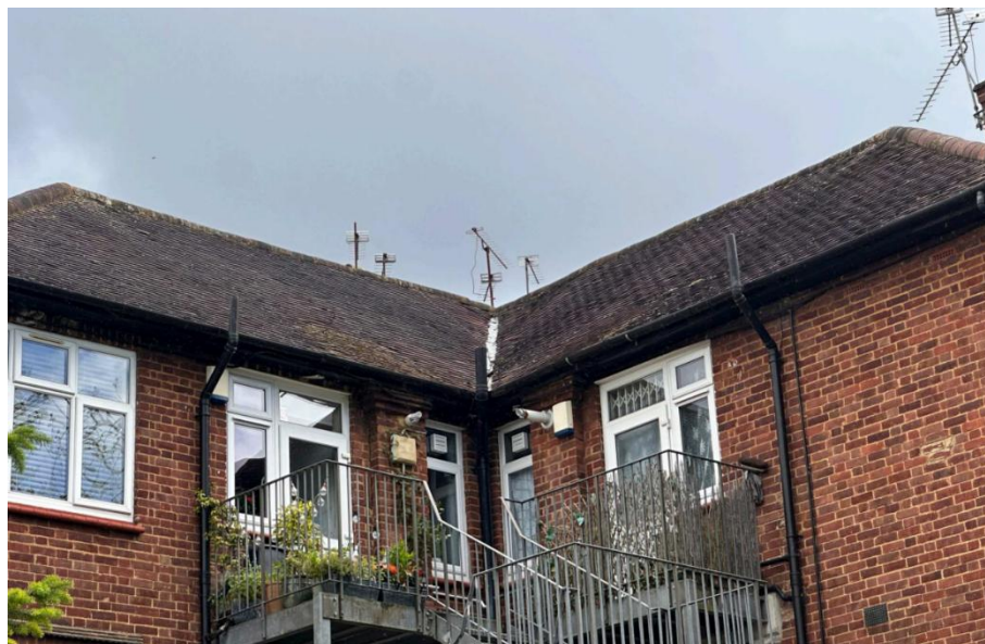
Photo 16 - Valley ridge on the south west aspect of the building with deteriorated mortar. (PRF10)
