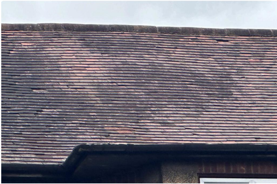
Photo 7 - Multiple displaced and lifted tiles. (PRF 1)
