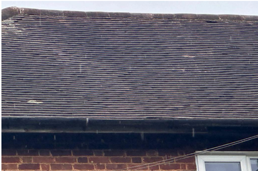
Photo 15 - Pitched roof with missing and slipped tiles. (PRF9)
