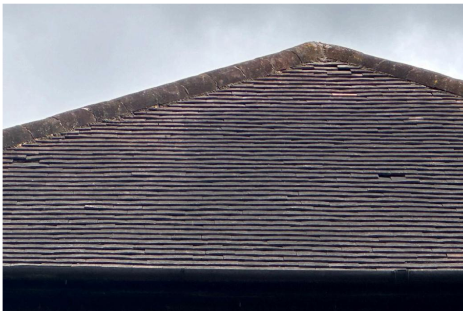
Photo 10 - Loose and partially displaced tiles (PRF4)
