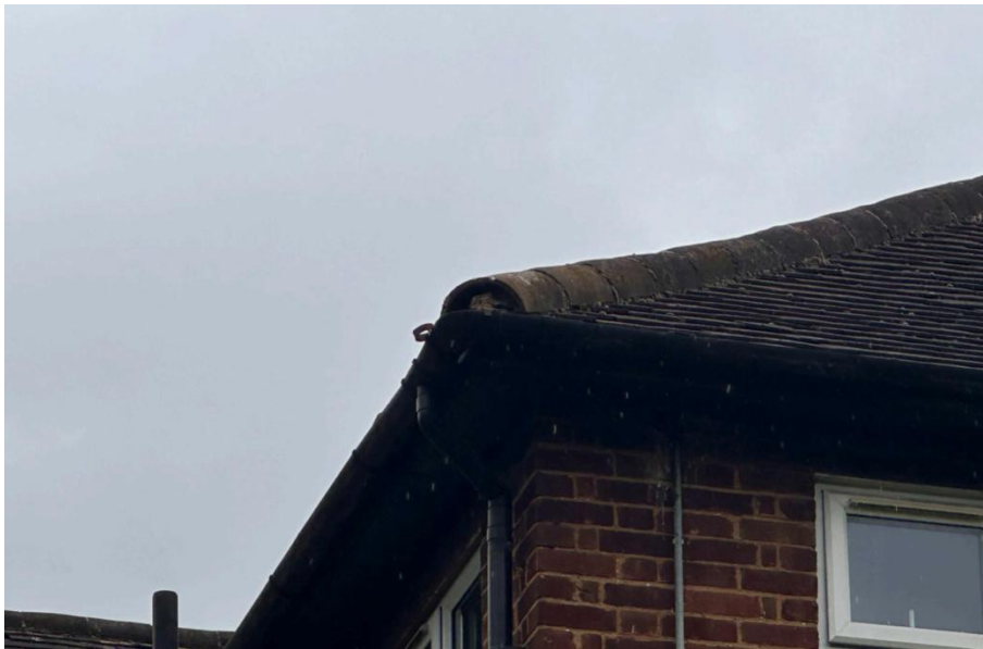
Photo 11 - Deteriorated hip mortar and gap at junction. (PRF5)
