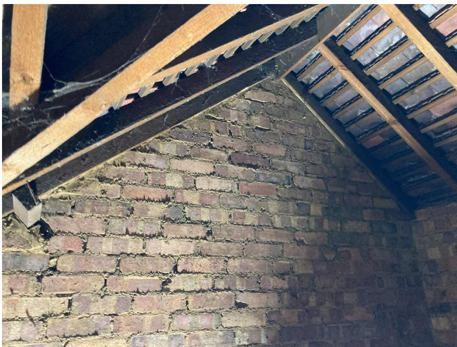
Photo 2 - Lack of insulation within roof void
