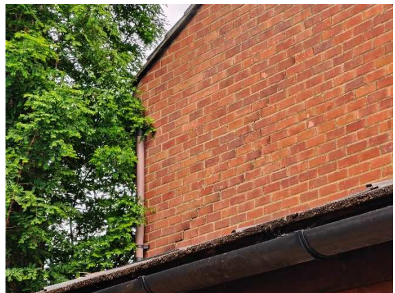
Fig 6: Cracks visible in brickwork on south-facing wall
