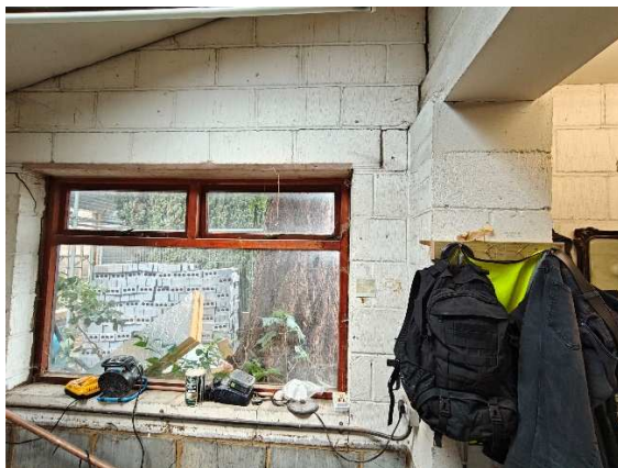
Fig 5: Cracks visible to blockwork inside the building
