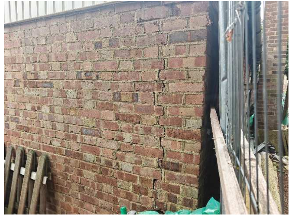
Fig 8: Cracks visible in brickwork
