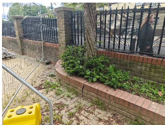
Fig 2: Crack adjacent to stem of hawthorn in small planter
