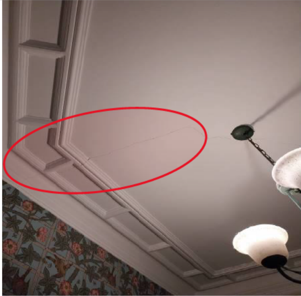
Photograph 4 – Entrance hallway cracking to ceiling
