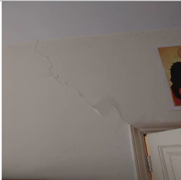
Photograph 6 – Cracking to Reception room 1
