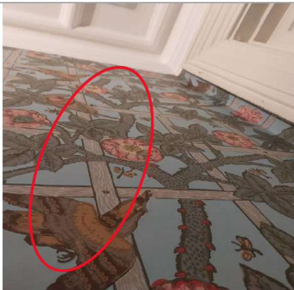
Photograph 3 - Diagonal cracking to hallway wall
