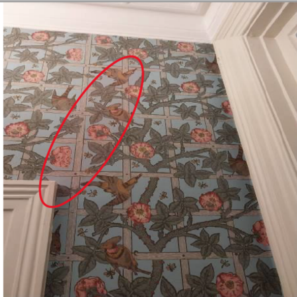
Photograph 2 – Diagonal cracking to hallway wall
