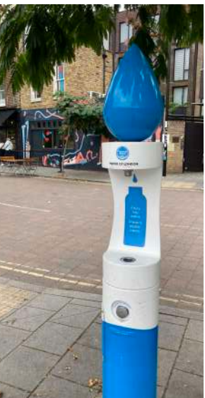
Drinking water fountain
