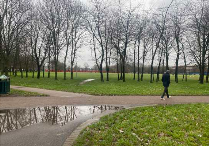
Pooling of water on existing hard-surfaces impedes pedestrian access
