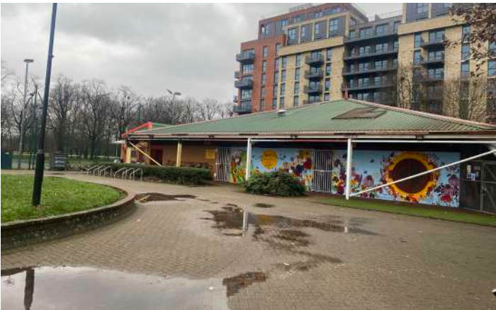
Pooling of water on surfaces in front of LUOS
