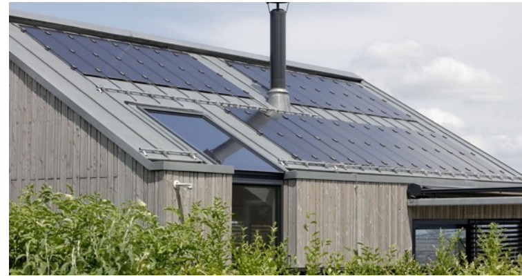
Example of roof mounted solar PV panels on a standing seam zinc roof © Rhienzink
