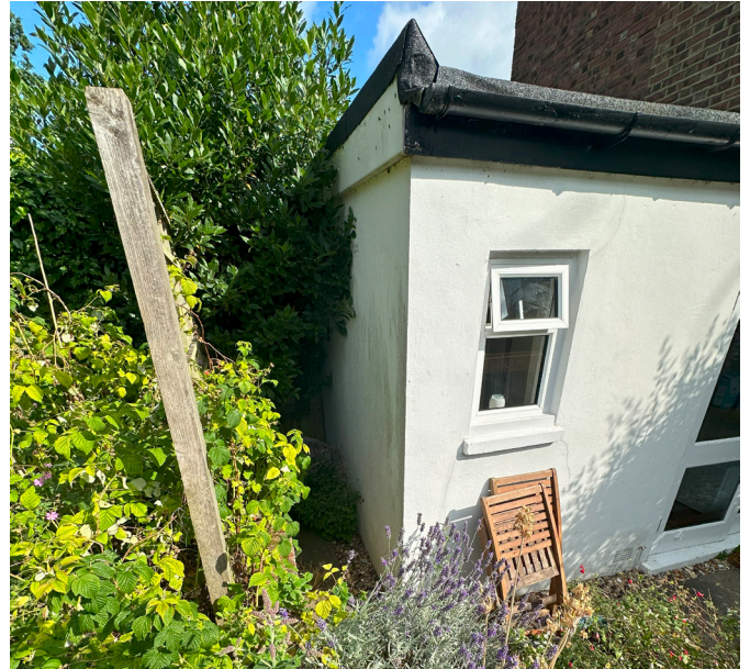
Existing Extension Condition
