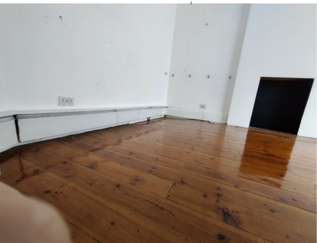
70MM SLOPE ACROSS LIVING ROOM FLOOR
