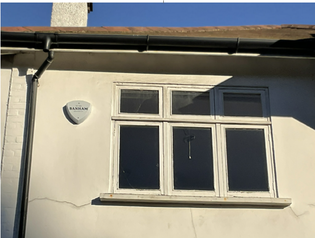
CRACKS IN SAND/ CEMENT RENDER TO EITHER SIDE AND BELOW WINDOW AT FRONT
