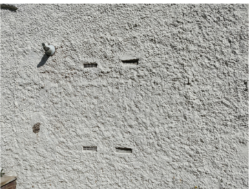
ROUGHCAST RENDER IS OVERLY THICK IN PARTS, UNEVEN AND PATCHY IN APPEARANCE AND IS GENERALLY IN A POOR CONDITION
