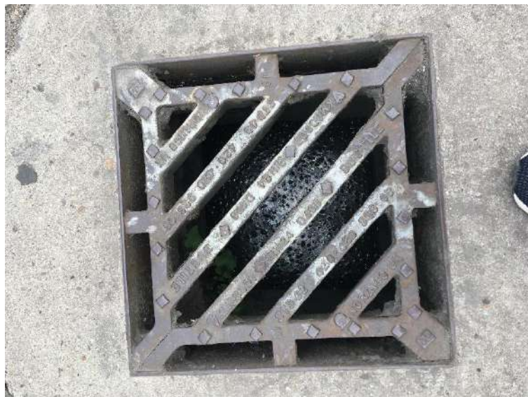
Photograph 10 – Drainage with potential petroleum product on surface.
