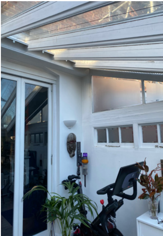
04 Internal view of conservatory and clerestory windows (single glazed roof and south facing aspect). The building currently over heats in summer.
