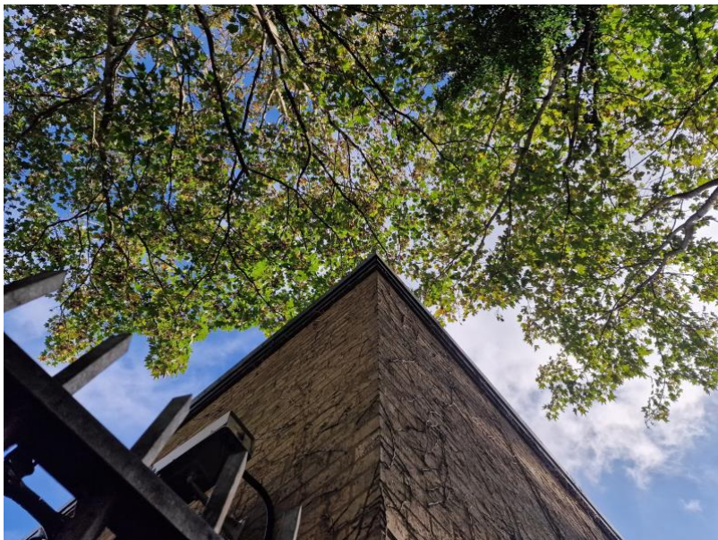
Figure 3: Upper crowns of T12 and T13 around 2.5 m clearance of the building's roof.
