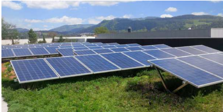
Figure 7: Example of angled PV system on a Green Roof
