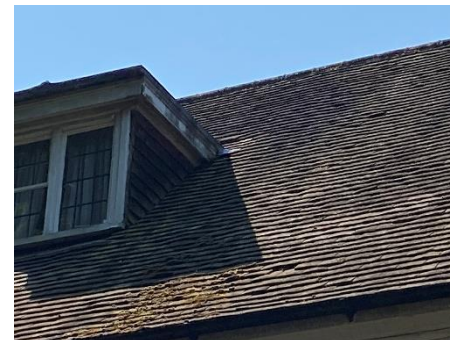
Figure 4: Missing, damaged and hanging tiles on adjoining building roof
