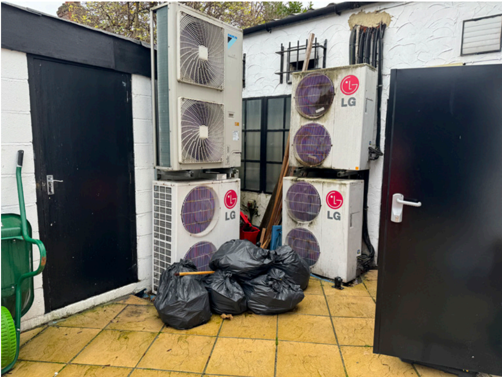
Above | 4no. ASHP + 1no. ASHP (behind, see drawing 0040_010 Ground Floor Plans_P1) in the Courtyard | 27/11/23
