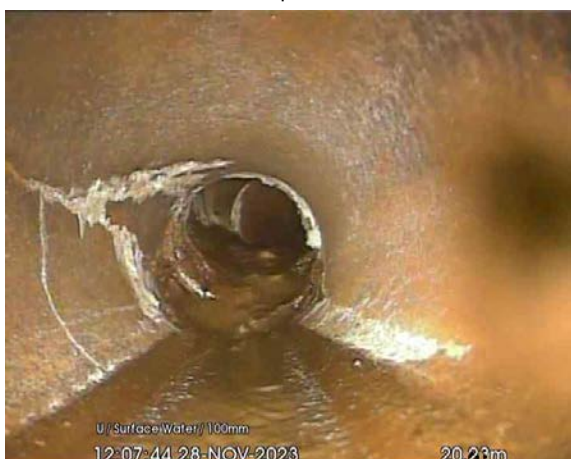
8-1-28A, 00:02:44, 20.23 m Cracks, multiple from 7 o'clock to 12 o'clock, start
