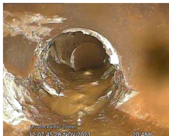
8-1-30A, 00:02:45, 20.48 m Joint displaced, large
