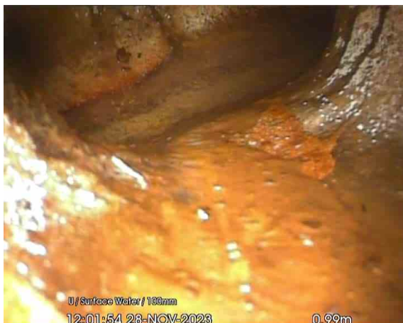
8-1-5A, 00:00:17, 0.99 m General remark, At junction to line from SWG1 downstream (point A1)
