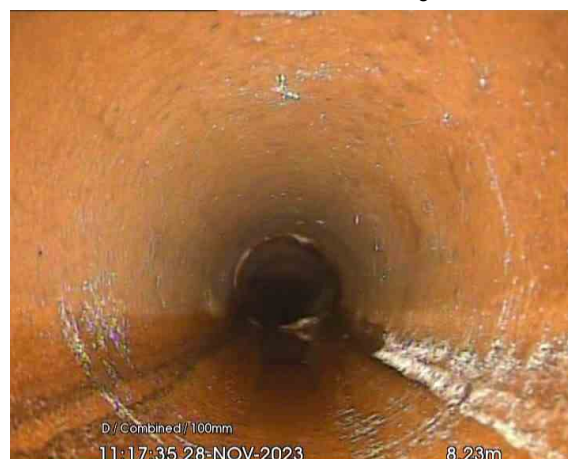
5-1-5A, 00:01:17, 8.23 m Crack, circumferential from 2 o'clock to 8 o'clock, Hairline crack
