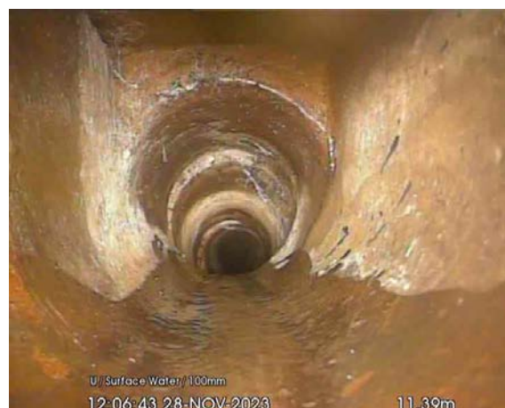
8-1-19A, 00:01:53, 11.39 m General remark, At access point in MH2 benching
