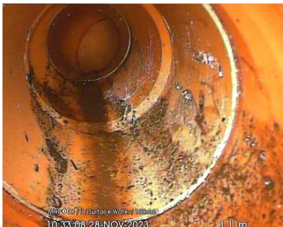
1-1-7A, 00:00:23, 1.11 m Junction at 10 o'clock, 100mm dia, from RWG2
