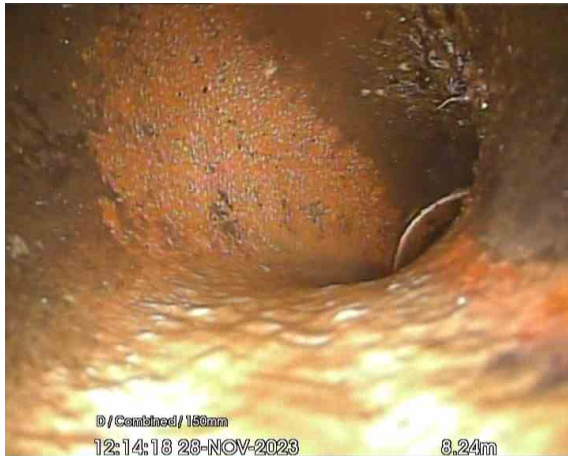
6-1-10A, 00:00:48, 8.24 m Line deviates right
