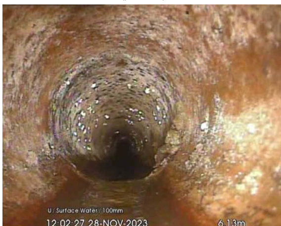
8-1-8A, 00:00:49, 6.13 m Attached deposits, other at joint from 3 o'clock to 5 o'clock, 10% cross-sectional area loss, Jointing intrusions/scale
