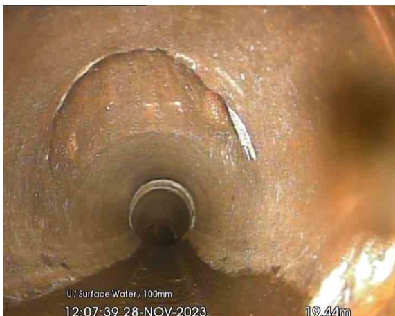
8-1-25A, 00:02:39, 19.44 m Junction at 11 o'clock, 100mm dia, H - not sourced / assumed lamphole
