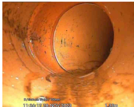
3-1-3A, 00:00:29, 1.33 m Line deviates right
