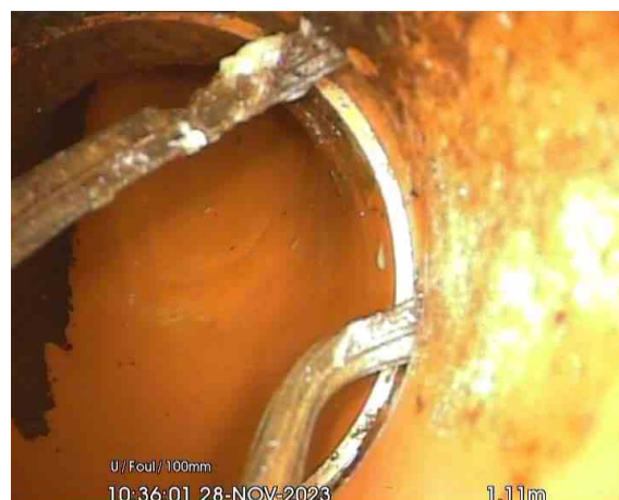
2-1-8A, 00:00:39, 1.11 m Sealing ring intruding from 12 o'clock to 12 o'clock
