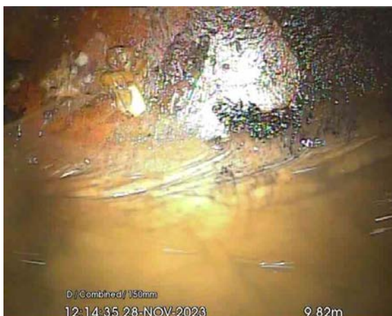
6-1-15A, 00:01:06, 9.82 m Finish node, other special chamber, reference: Main FW Sewer, At Main FW Sewer
