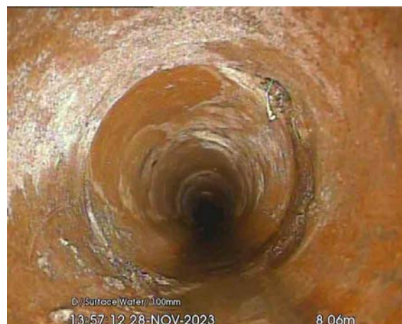
7-1-8A, 00:01:33, 8.06 m Joint displaced, medium
