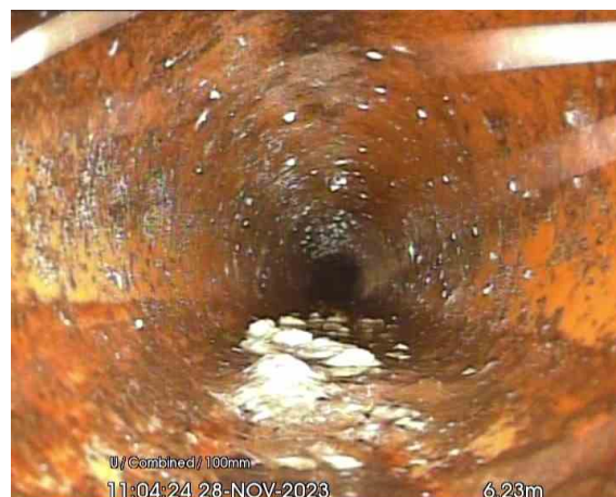
4-1-8A, 00:01:13, 6.23 m Settled deposits, other, 10% cross-sectional area loss, start, Debris/waste
