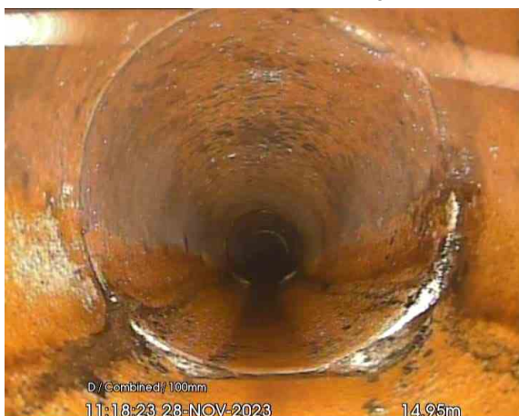
5-1-7A, 00:02:06, 14.95 m Joint displaced, medium
