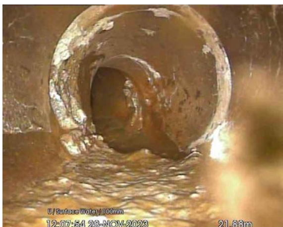
8-1-32A, 00:02:54, 21.88 m Attached deposits, encrustation at joint from 12 o'clock to 12 o'clock, 10% cross-sectional area loss, Jointing
