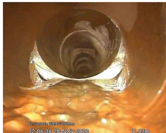
8-1-15A, 00:01:46, 11.03 m Joint displaced, large
