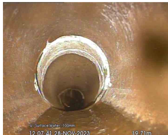
8-1-26A, 00:02:41, 19.71 m Joint displaced, medium
