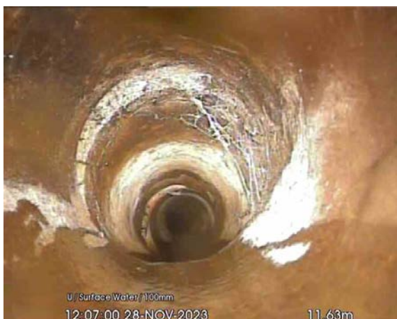
8-1-22A, 00:02:00, 11.63 m Joint displaced, medium
