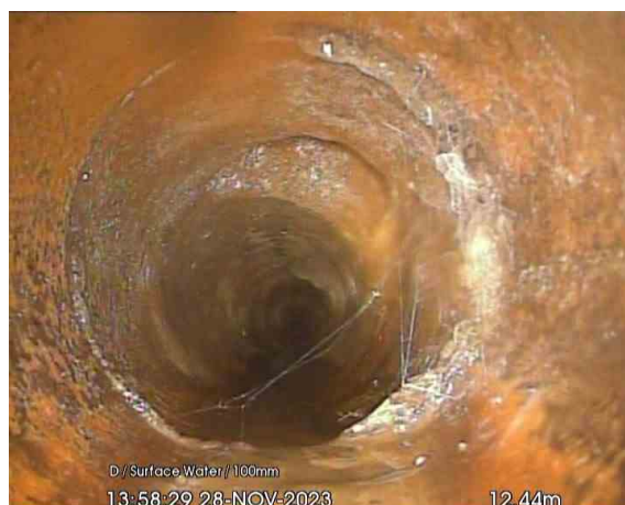
7-1-14A, 00:02:36, 12.44 m Attached deposits, other at joint from 12 o'clock to 6 o'clock, 5% cross-sectional area loss, Jointing intrusions
