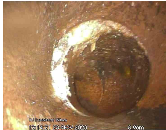
6-1-11A, 00:00:52, 8.96 m Joint displaced, medium
