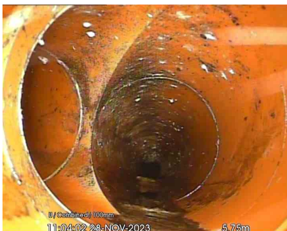
4-1-7A, 00:01:06, 5.75 m Junction at 9 o'clock, 100mm dia, B - not sourced / assumed from WC
