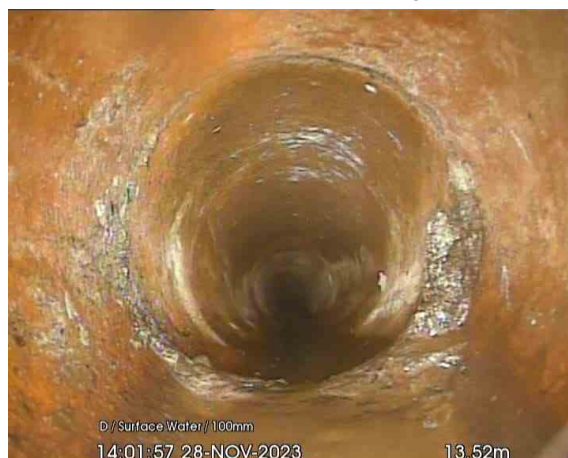
7-1-16A, 00:02:57, 13.52 m Attached deposits, other at joint from 3 o'clock to 8 o'clock, 10% cross-sectional area loss, Jointing intrusions
