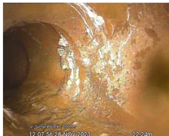
8-1-34A, 00:02:56, 22.24 m General remark, Approaching junction to Main SW Sewer in Grove Avenue
