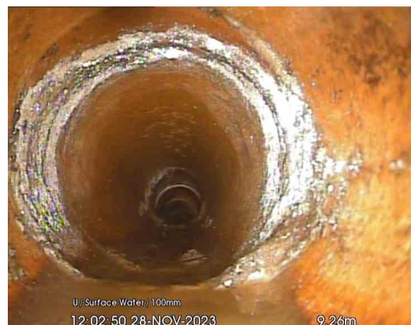
8-1-9A, 00:01:12, 9.26 m Settled deposits, other at joint, 10% cross-sectional area loss, Jointing intrusions/scale
