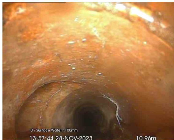
7-1-11A, 00:02:04, 10.96 m Junction at 10 o'clock, 100mm dia, F - not sourced/possible from No.71
