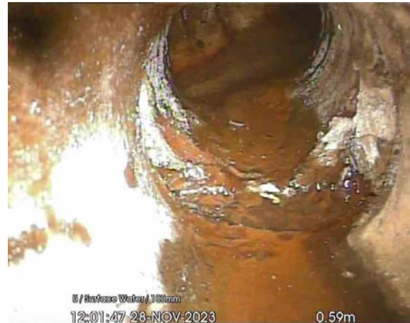
8-1-4A, 00:00:10, 0.59 m Joint displaced, large
