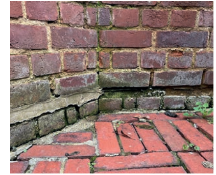
DPC level compromised
