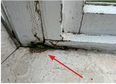
Thermal Bridges + Leaky Interfaces
