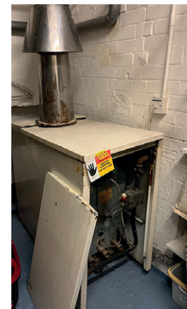
Condemned Heating System
