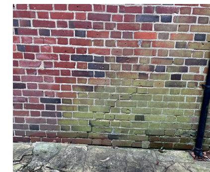
Structural Cracking in wall
