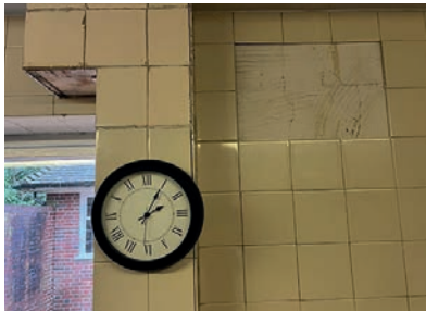
Unsuitable surface condition
