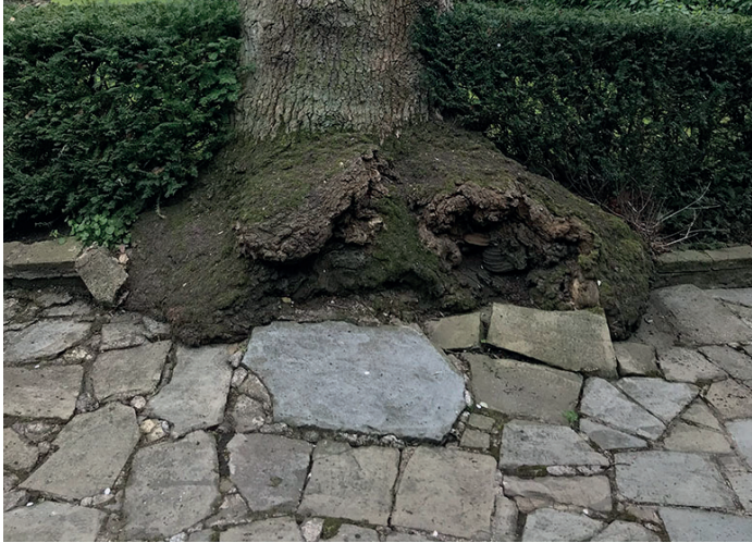
Pavement obstructs tree growth, damaging both tree and pavement
