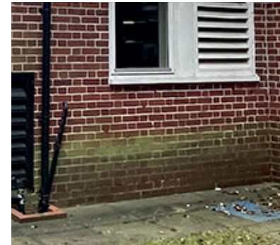
Rising Damp wet base + moss
