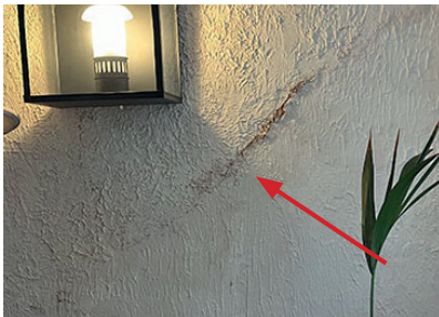
Moisture penetrating through wall
