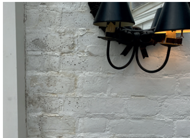
Surface condensation; mould growth
