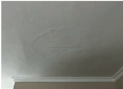
Moisture penetrating through ceiling
