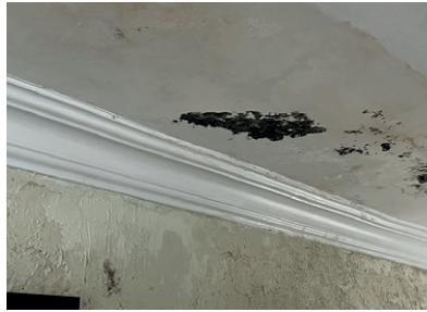
Ceiling - more black mould
