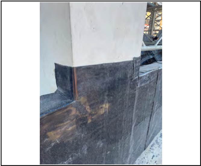
Sealed column detailing.
