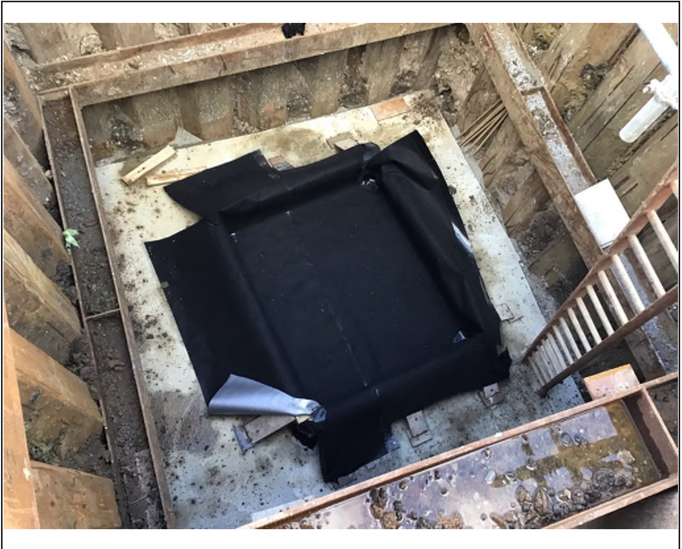
Pump Chamber Base
