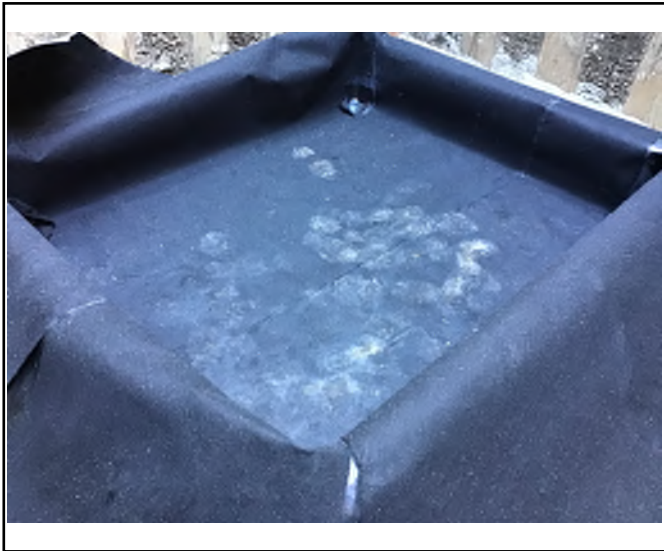
Pump chamber base tested with
