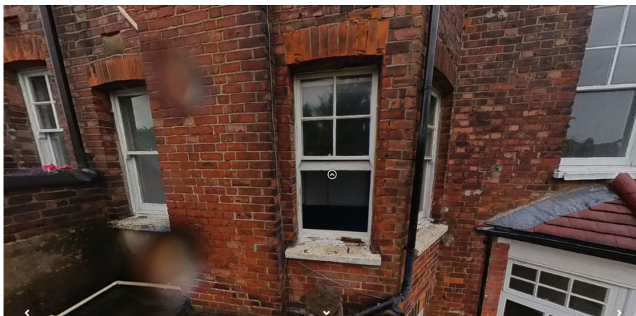
Above – Photographs of state of repair of existing windows in front (top) and rear (bottom).
