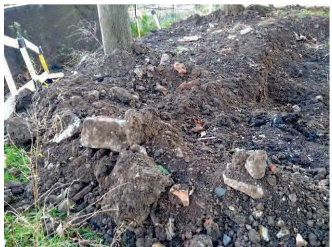
Plate 12: Made Ground/spoil from the repair of the gas main.
