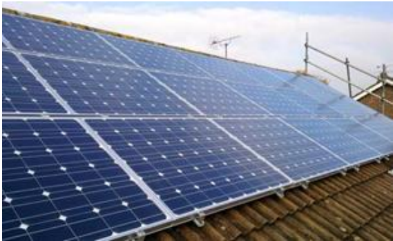
Figure 6: Roof Mounted PV Panels
