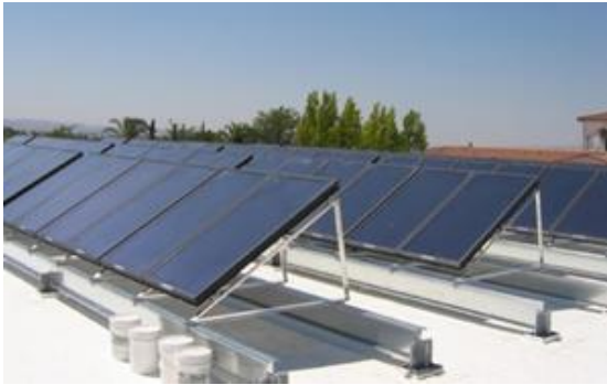
Figure 7: Frame Mounted PV Panels
