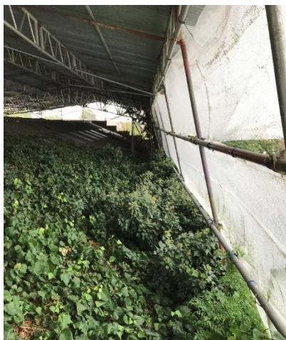
Damaged existing roof and temporary roof structure
