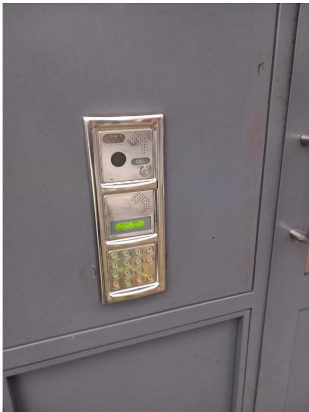
Door entry Panel (to be replaced)
