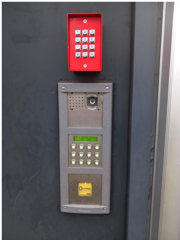
Door entry Panel (to be replaced)
