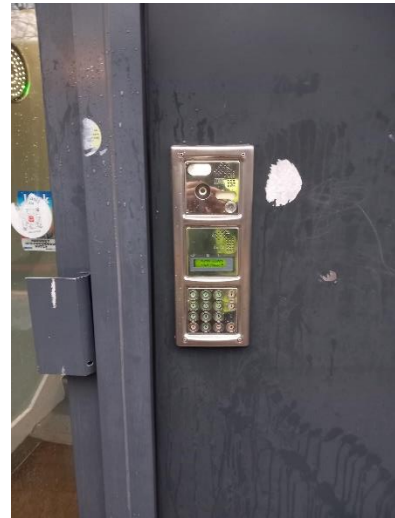
Door entry Panel (to be replaced)
