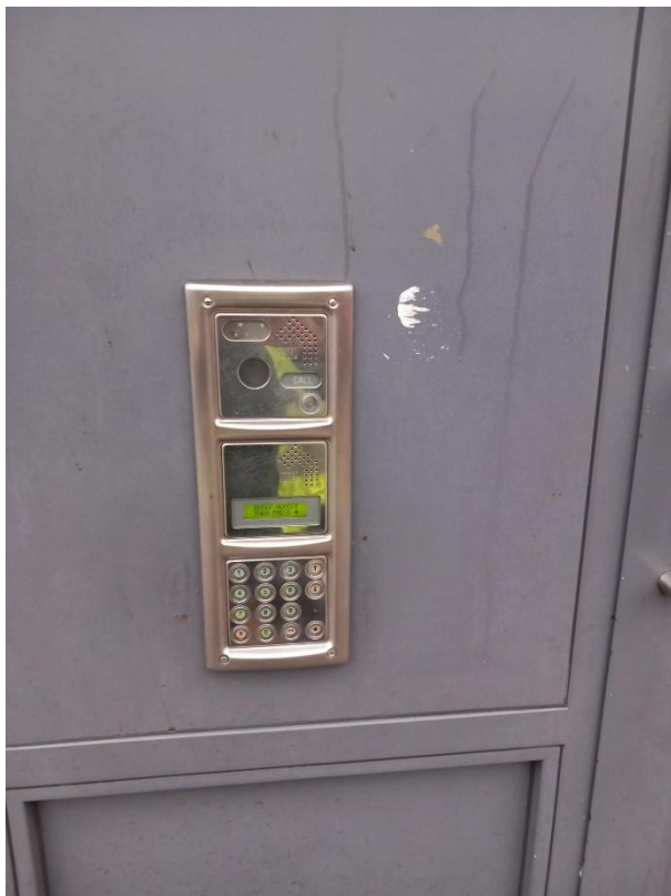
Door entry Panel (to be replaced)
