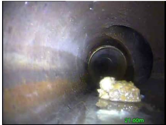
10, 00:01:55, 21.60 m Junction at 2 o'clock, 100mm dia
