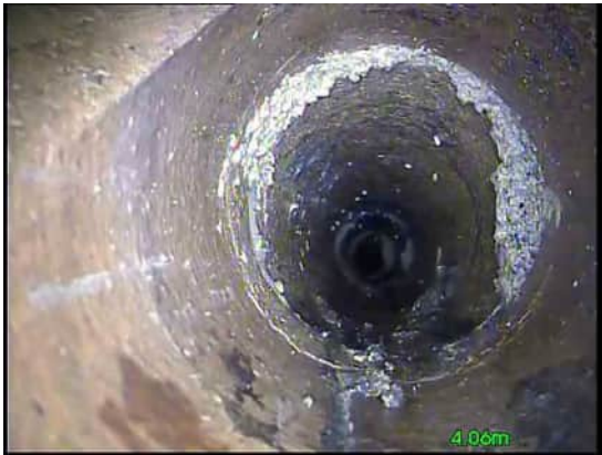
6, 00:00:35, 4.06 m Settled deposits, fine at joint, 5% cross-sectional area loss
