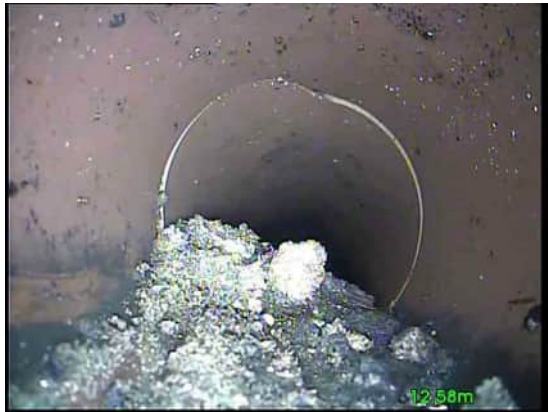
6, 00:00:50, 12.58 m Settled deposits, coarse, 35% cross-sectional area loss, change
