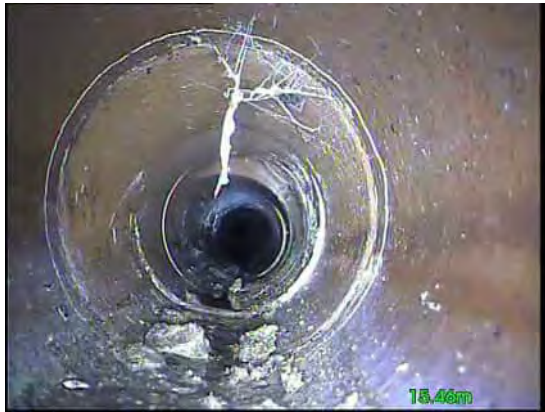
13, 00:01:44, 15.46 m Crack, circumferential at joint from 8 o'clock to 4 o'clock
