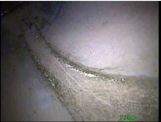
8, 00:00:39, 7.31 m General remark, Sewer levels out at this point
