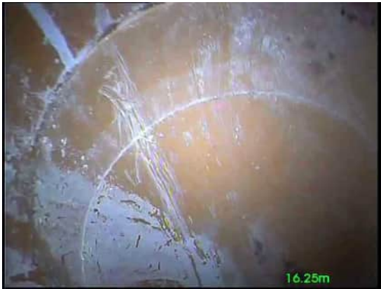
6, 00:00:47, 16.25 m General remark, Sewer levels out at this point
