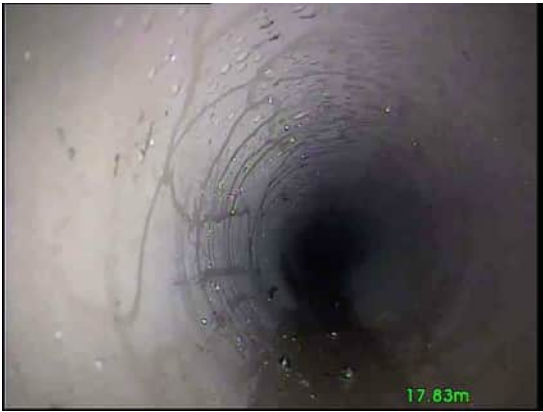
19, 00:02:08, 17.83 m Pipe material changes to polyvinyl chloride at this point
