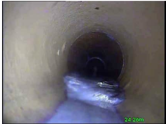
12, 00:03:53, 24.26 m Settled deposits, hard or compacted, 10% cross-sectional area loss, start
