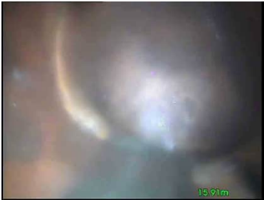
14, 00:09:07, 15.91 m Line deviates down, At entry to main public sewer
