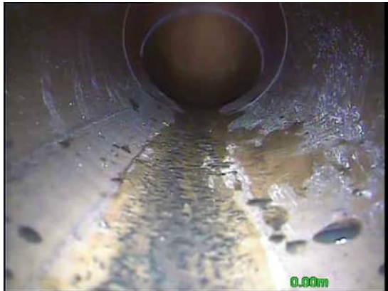
1, 00:00:02, 0.00 m Line deviates up
