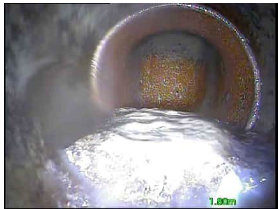
4, 00:00:22, 1.80 m Finish node, other special chamber, reference: Downpipe, Internal downpipe reached
