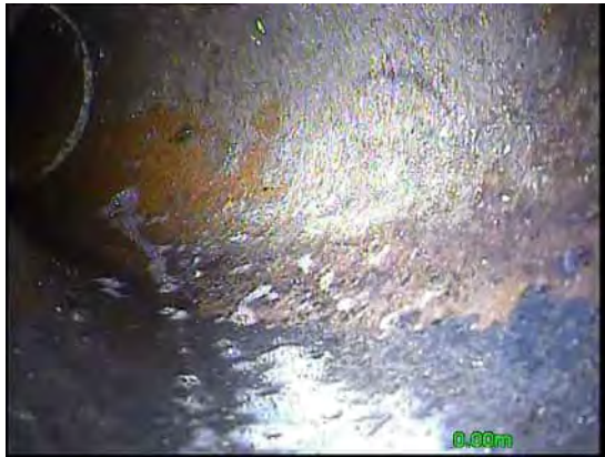
1, 00:00:02, 0.00 m Line deviates up
