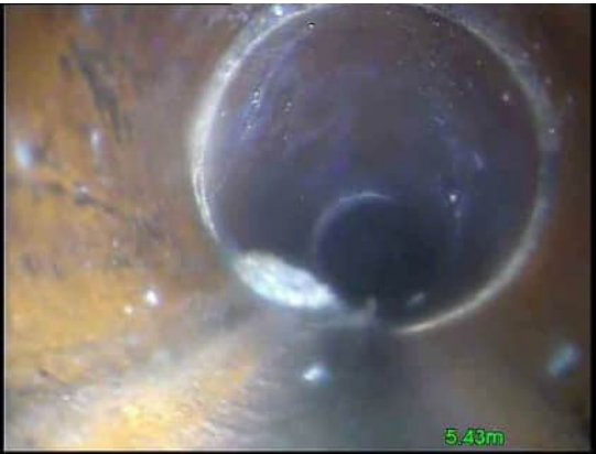
6, 00:02:48, 5.43 m Settled deposits, hard or compacted at joint, 5% cross-sectional area loss
