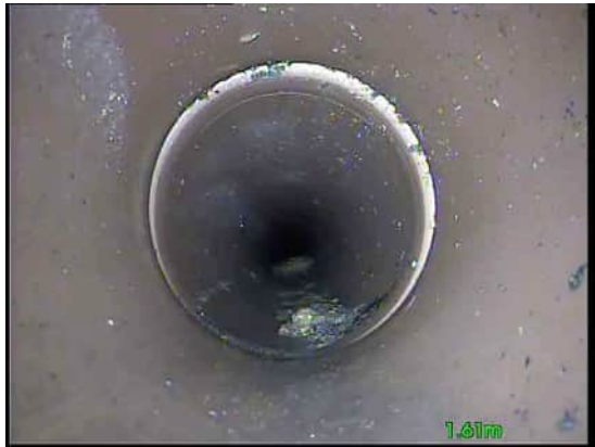
2, 00:00:10, 1.61 m Crack, circumferential at joint from 10 o'clock to 2 o'clock
