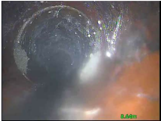
9, 00:05:13, 8.64 m Settled deposits, fine at joint, 5% cross-sectional area loss
