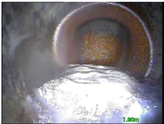
3, 00:00:22, 1.80 m Settled deposits, hard or compacted, 20% cross-sectional area loss, At rest bend of downpipe
