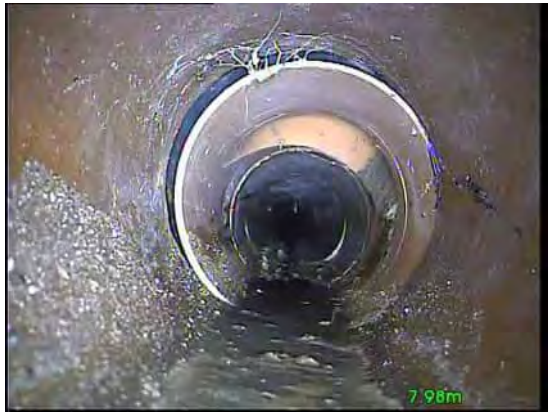
5, 00:00:48, 7.98 m Pipe material changes to polyvinyl chloride at this point
