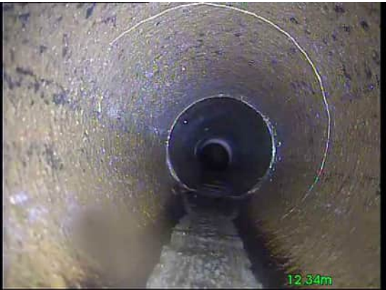
8, 00:01:00, 12.34 m Crack, circumferential from 10 o'clock to 4 o'clock
