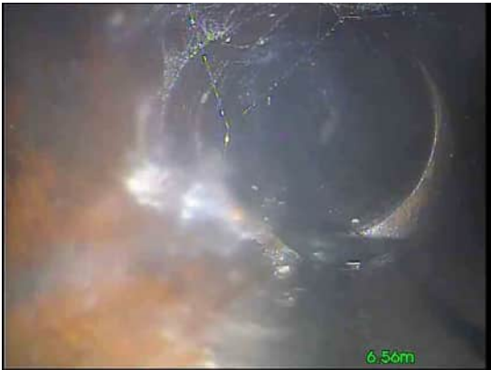
7, 00:05:01, 6.56 m Joint displaced, large
