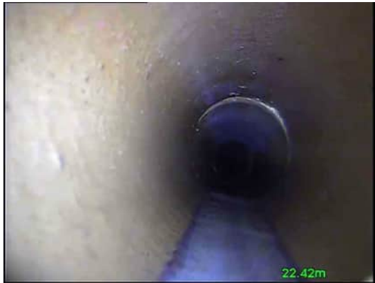
11, 00:02:18, 22.42 m Attached deposits, fouling from 5 o'clock to 7 o'clock, 5% cross-sectional area loss, finish
