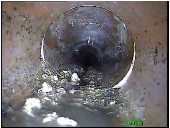
8, 00:00:56, 8.40 m Settled deposits, coarse, 5% cross-sectional area loss, start
