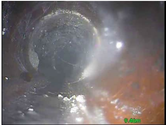
11, 00:05:30, 9.46 m Settled deposits, fine at joint, 5% cross-sectional area loss
