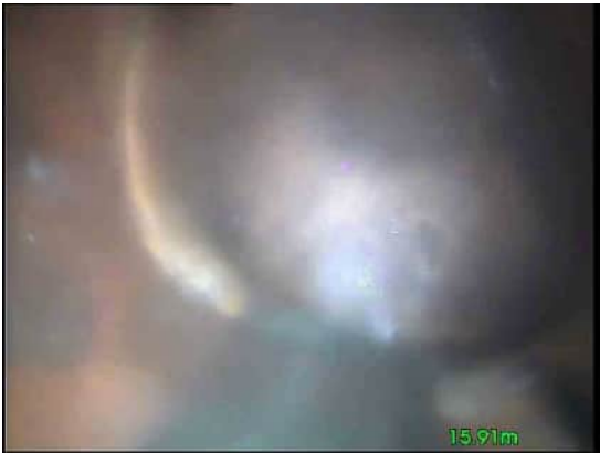
15, 00:09:07, 15.91 m Finish node, major connection without manhole, reference: Main public sewer reached
