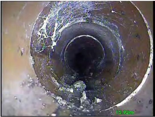
16, 00:01:55, 15.92 m Pipe material changes to vitrified clay at this point
