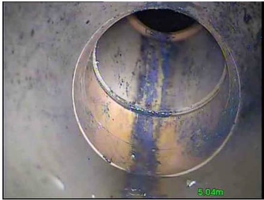
3, 00:00:33, 5.04 m Line deviates up
