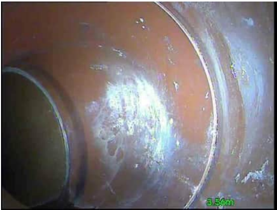
5, 00:00:17, 3.56 m Line deviates down
