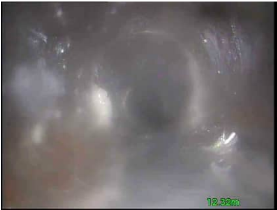
13, 00:09:32, 12.32 m Settled deposits, fine at joint, 5% cross-sectional area loss
