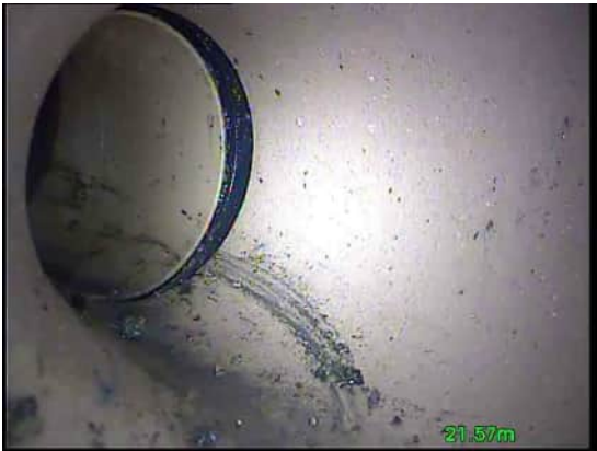
22, 00:02:27, 21.57 m Line deviates up
