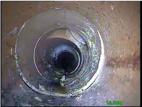
14, 00:01:50, 15.54 m Pipe material changes to polyvinyl chloride at this point
