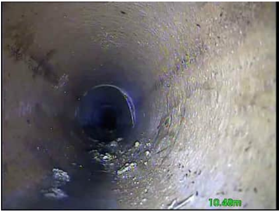
11, 00:01:16, 10.48 m Settled deposits, coarse, 5% cross-sectional area loss, start
