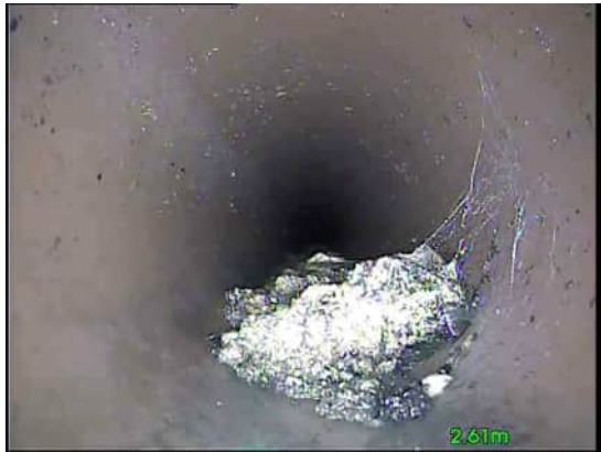
3, 00:00:14, 2.61 m Settled deposits, coarse, 20% cross-sectional area loss, start
