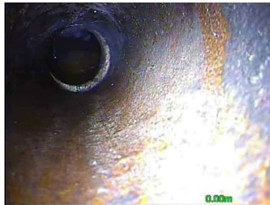
1, 00:00:02, 0.00 m Line deviates up
