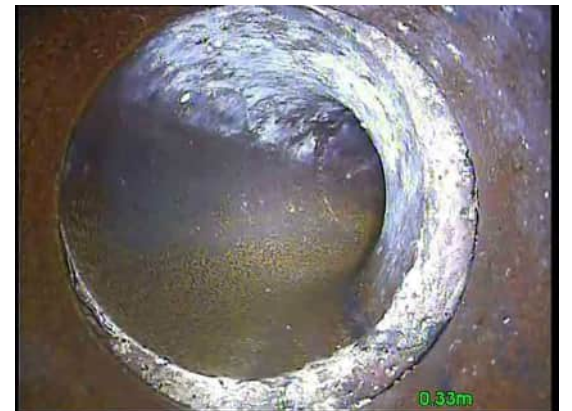
2, 00:00:08, 0.33 m Joint displaced, medium
