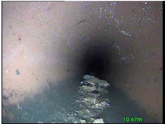
5, 00:00:41, 10.67 m Settled deposits, coarse, 10% cross-sectional area loss, start
