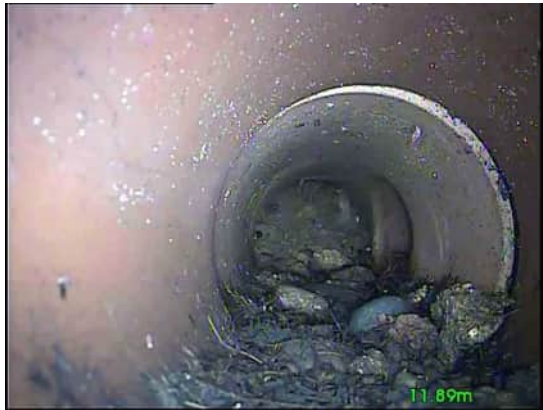
7, 00:00:46, 11.89 m Settled deposits, coarse, 25% cross-sectional area loss, start
