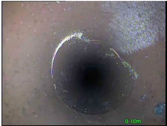
1, 00:00:03, 0.10 m Fracture, circumferential from 9 o'clock to 11 o'clock
