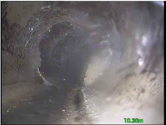
12, 00:05:34, 10.30 m Settled deposits, fine at joint, 5% cross-sectional area loss
