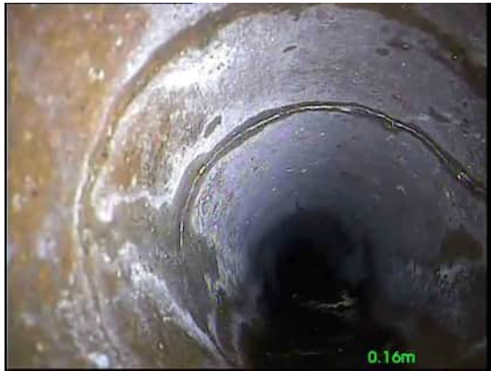
1, 00:00:03, 0.16 m Crack, circumferential from 9 o'clock to 3 o'clock
