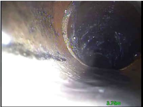
4, 00:01:03, 3.75 m Line deviates down
