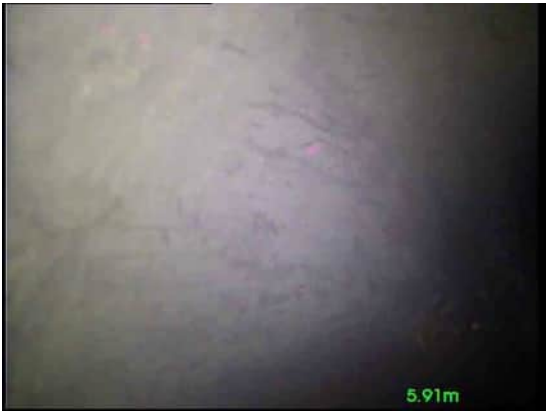
4, 00:00:28, 5.91 m General remark, Sewer levels out at entry to MH9
