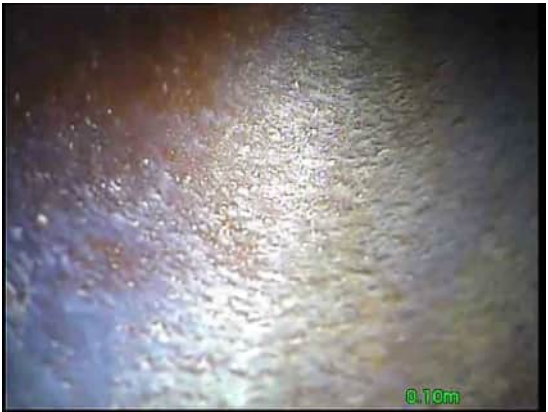
2, 00:00:05, 0.10 m Line deviates up
