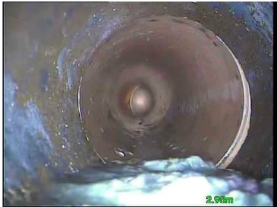
3, 00:00:26, 2.95 m Attached deposits, fouling from 5 o'clock to 7 o'clock, 5% cross-sectional area loss
