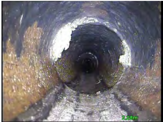
4, 00:00:20, 2.28 m Settled deposits, fine at joint, 5% cross-sectional area loss
