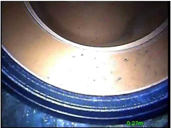
2, 00:00:13, 0.27 m Pipe material changes to polyvinyl chloride at this point
