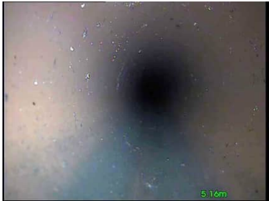
4, 00:00:25, 5.16 m Settled deposits, coarse, 20% cross-sectional area loss, finish
