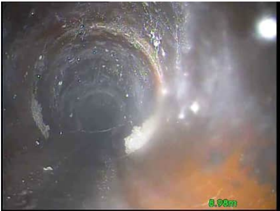
10, 00:05:18, 8.98 m Settled deposits, fine at joint, 5% cross-sectional area loss
