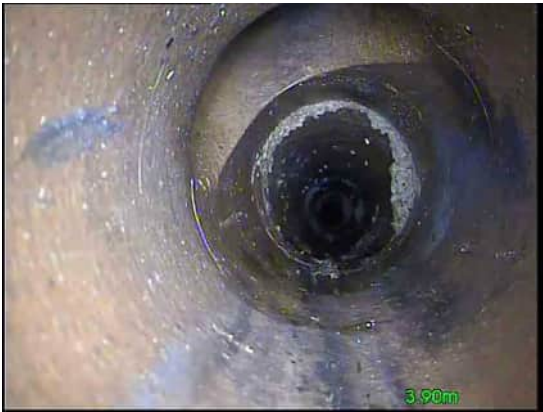
5, 00:00:30, 3.90 m Junction at 11 o'clock, 100mm dia
