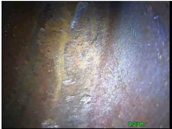
1, 00:00:10, 0.23 m Line deviates up
