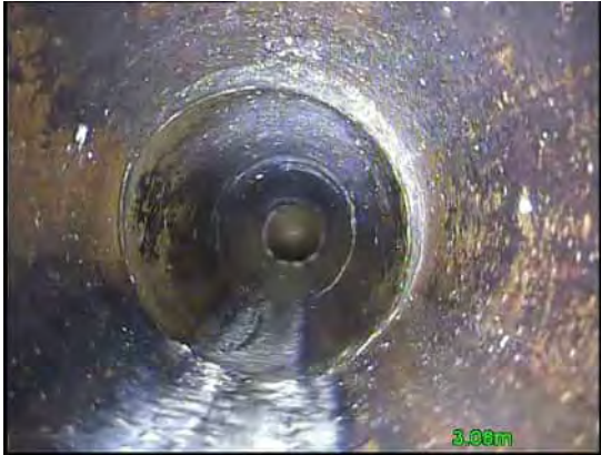
2, 00:00:13, 3.08 m Line deviates up
