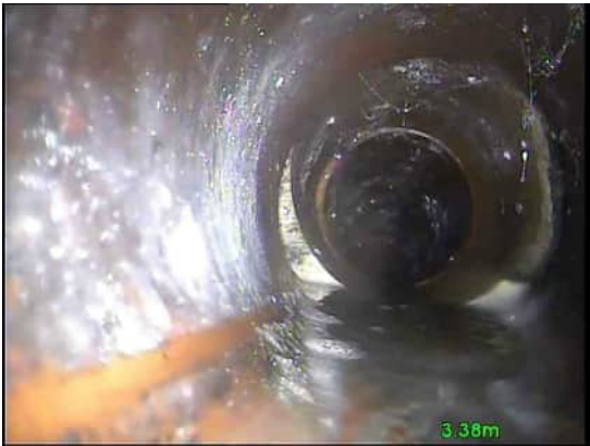
3, 00:00:51, 3.38 m Joint displaced, large
