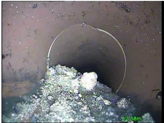
7, 00:00:50, 12.58 m Fracture, circumferential from 12 o'clock to 12 o'clock
