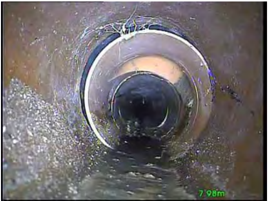
6, 00:00:48, 7.98 m Joint displaced, medium
