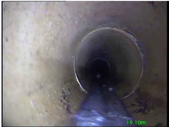
8, 00:01:36, 19.10 m Attached deposits, fouling from 4 o'clock to 8 o'clock, 10% cross-sectional area loss, finish
