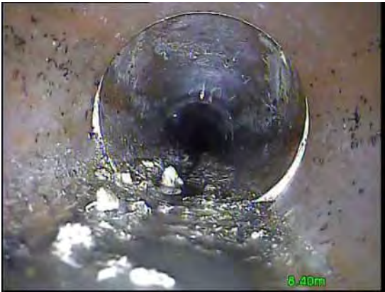
9, 00:00:56, 8.40 m Pipe material changes to vitrified clay at this point
