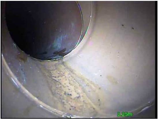
4, 00:00:24, 3.25 m Line deviates up
