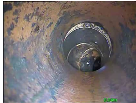
1, 00:00:03, 0.04 m Line deviates up
