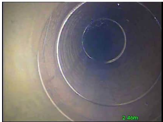
4, 00:00:18, 2.46 m General remark, Sewer levels out at this point
