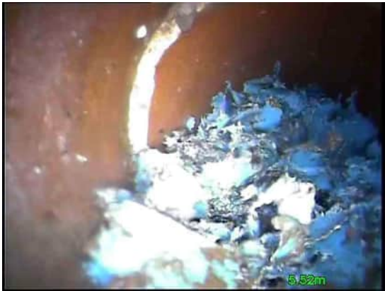
6, 00:00:39, 5.52 m Settled deposits, other, 100% cross-sectional area loss, Pipe full of loose plastic
