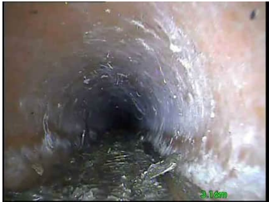
2, 00:00:14, 3.16 m Settled deposits, fine, 10% cross-sectional area loss, finish
