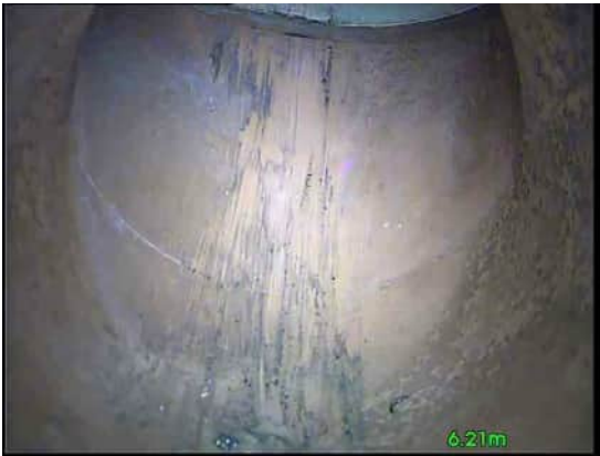
5, 00:00:37, 6.21 m Finish node, other special chamber, reference: RWP, Internal RWP reached
