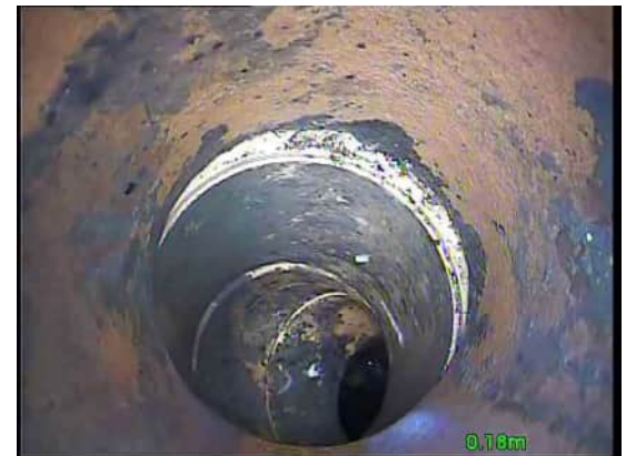
2, 00:00:06, 0.18 m Pipe material changes to polyvinyl chloride at this point
