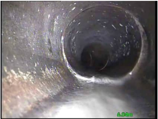
6, 00:00:41, 6.04 m Joint displaced, medium
