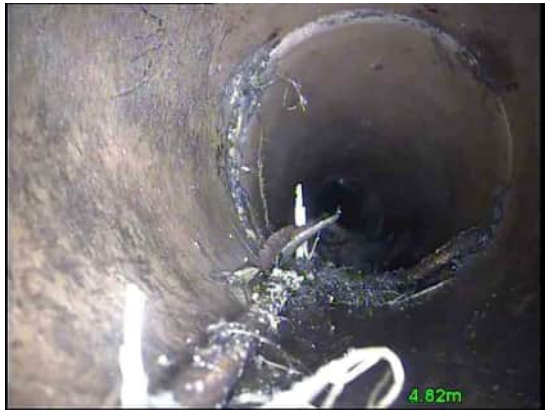
7, 00:00:45, 4.82 m Roots, tap at joint
