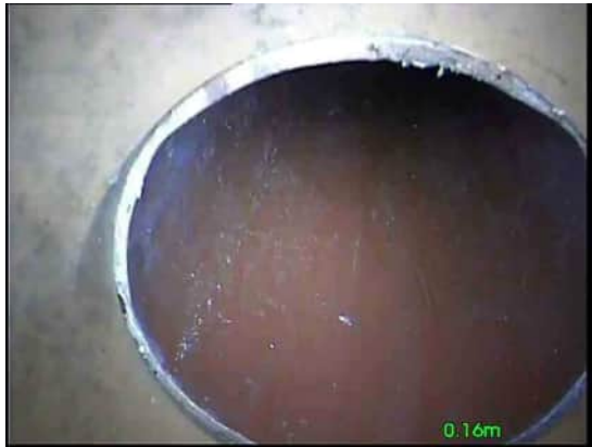
1, 00:00:04, 0.16 m Line deviates up
