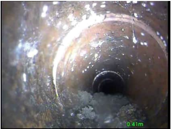
2, 00:00:05, 0.41 m Settled deposits, fine, 25% cross-sectional area loss, start
