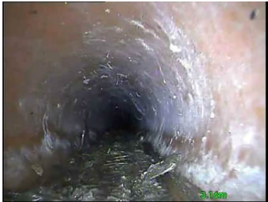
3, 00:00:14, 3.16 m Settled deposits, coarse, 10% cross-sectional area loss, start
