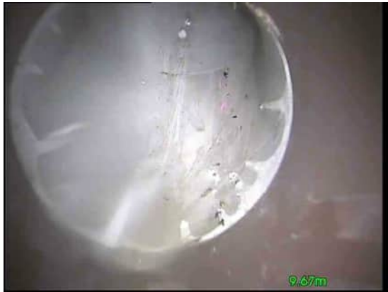
9, 00:01:23, 9.67 m Finish node, other special chamber, reference: RWP, Internal RWP reached
