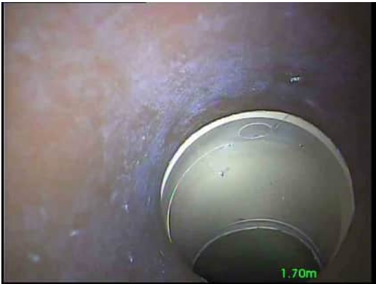
2, 00:00:11, 1.70 m General remark, Sewer levels out at this point
