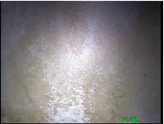
10, 00:01:20, 12.54 m Finish node, other special chamber, reference: RWP, Internal RWP reached
