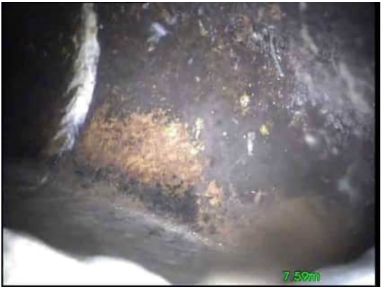
9, 00:00:50, 7.59 m Finish node, major connection without manhole, reference: Main public sewer reached
