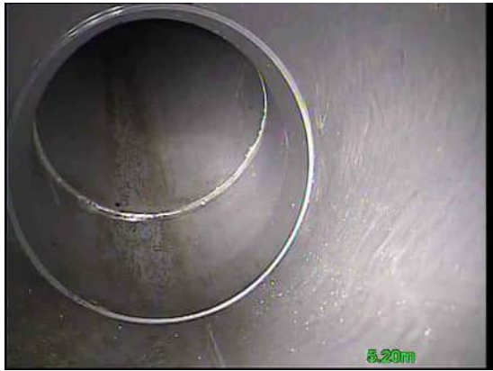
7, 00:00:46, 5.20 m Line deviates up
