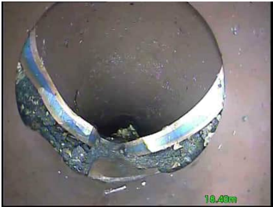
6, 00:01:09, 18.40 m Joint displaced, large
