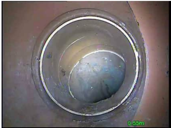
2, 00:00:11, 0.55 m Line deviates up
