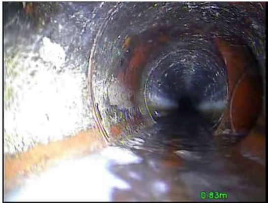
1, 00:00:10, 0.83 m Junction at 3 o'clock, 100mm dia
