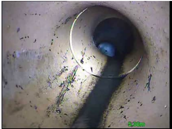
5, 00:00:33, 5.30 m Line deviates up
