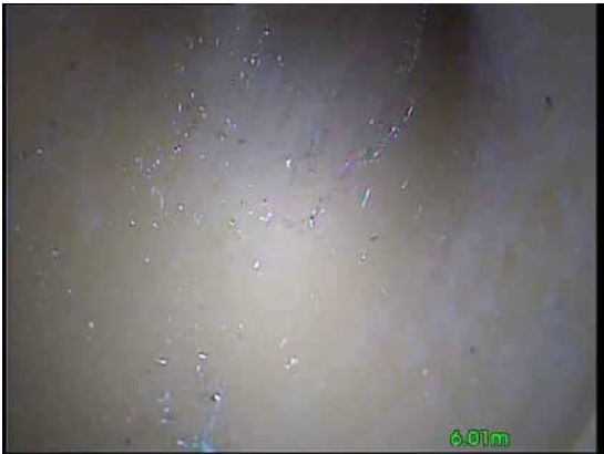
4, 00:00:26, 6.01 m Line deviates up
