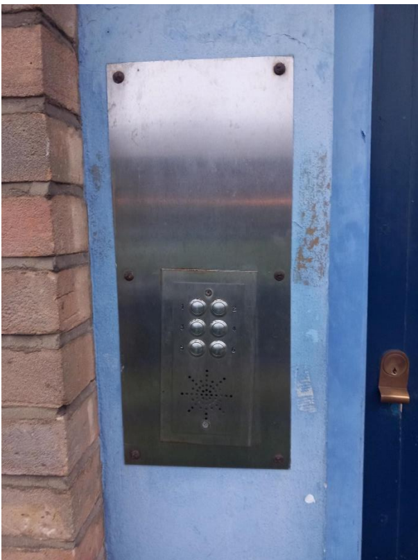
Door entry Panel (to be replaced)
