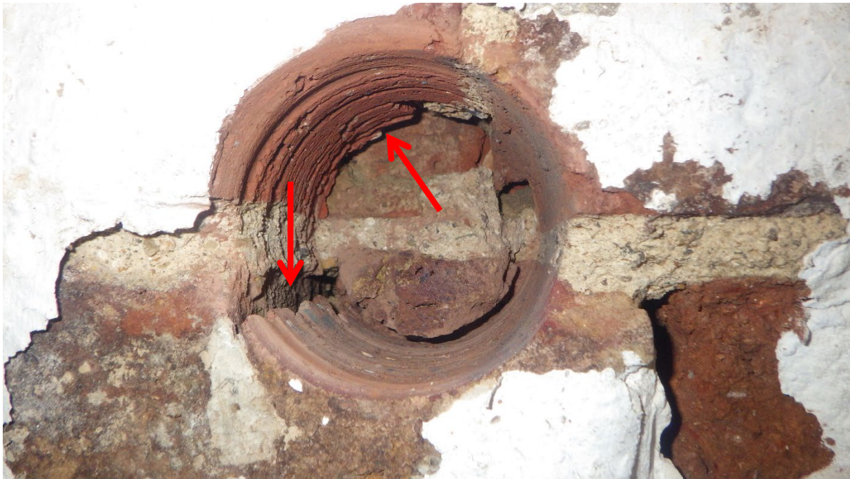
Photograph 12 Location C2. Vertical voids in joints to left and at towards back of hole.
