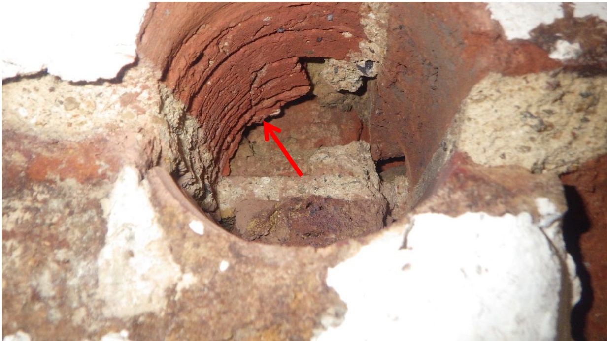
Photograph 14 Location C2. Vertical voids between bricks towards back of hole.
