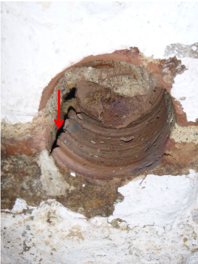
Photograph 13 Location C2. Vertical void between bricks on left.
