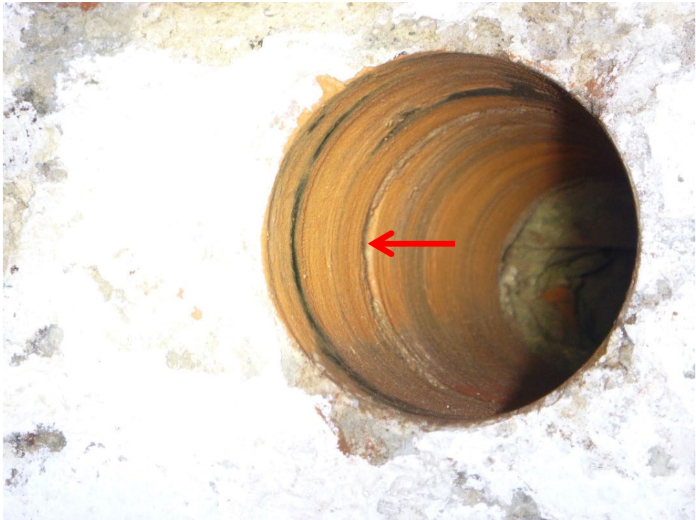
Photograph 4 Location A1. View of slight void in joint on left side of hole.
