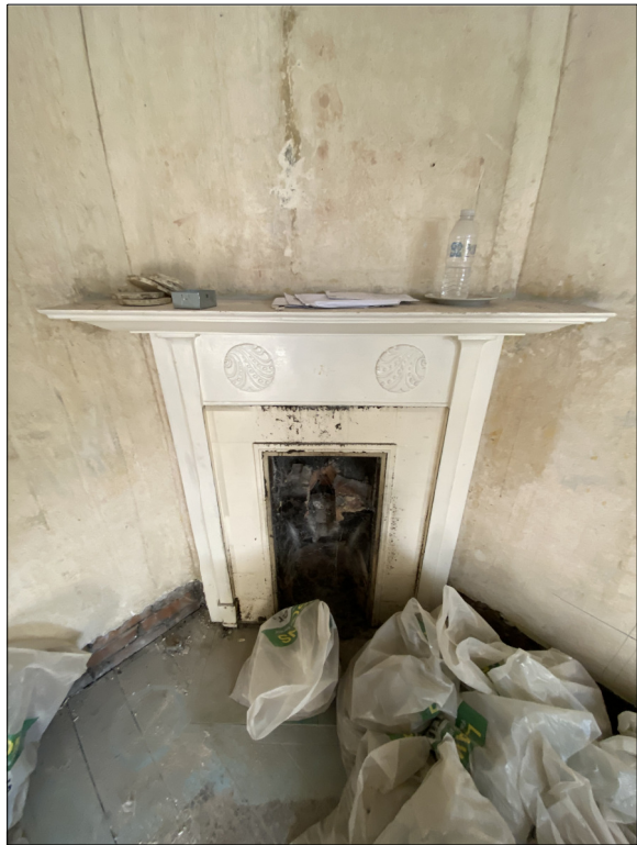
Fireplace 2 as existing Existing insert missing with fire proof backing damaged. Existing backing to remain on site with new tiles to conceal it.
