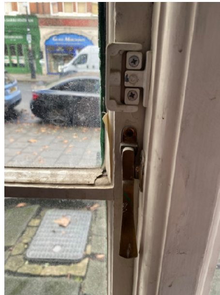
Poor quality historic alteration that will be replaced
