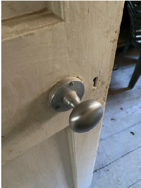
Poor quality internal door ironmongery to be replaced
