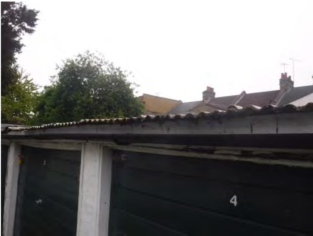
Further potential asbestos roofing on two of th
