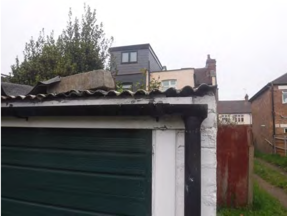
Potential asbestos roofing on the western garages. Access track on far right.
